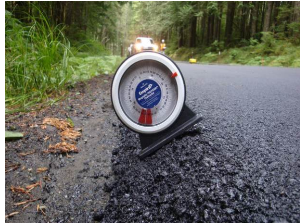
Figure 56. Slope indicator device on the edge treatment. Slope does not appear to be compacted.
