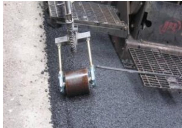
Figure 32. Roller added to compact the vertical edge at the top of the slope.
