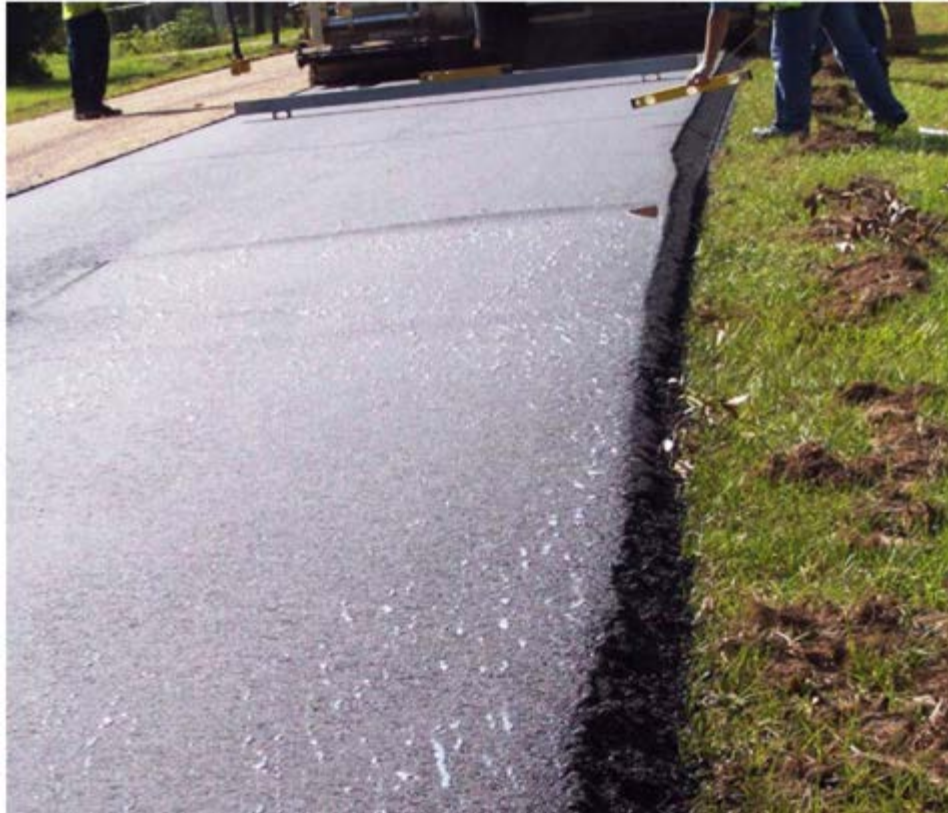
Figure 7. Pavement edge without the Safety Edge SM in foreground and with the Safety Edge SM in the background. (FHWA Safety Edge PowerPoint)
