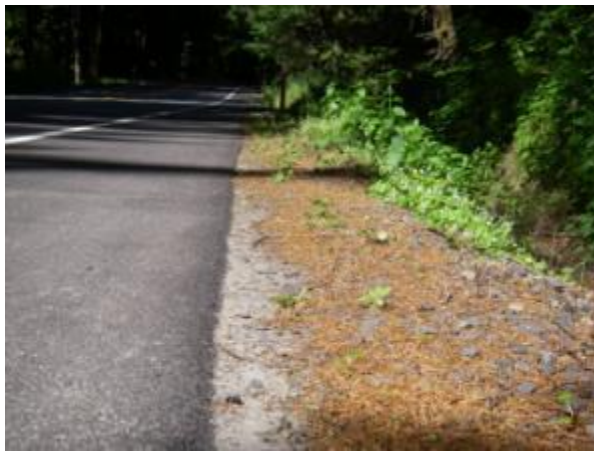
Figure 39. Another photo of the SR-410 pavement edge treatment one year after construction.
