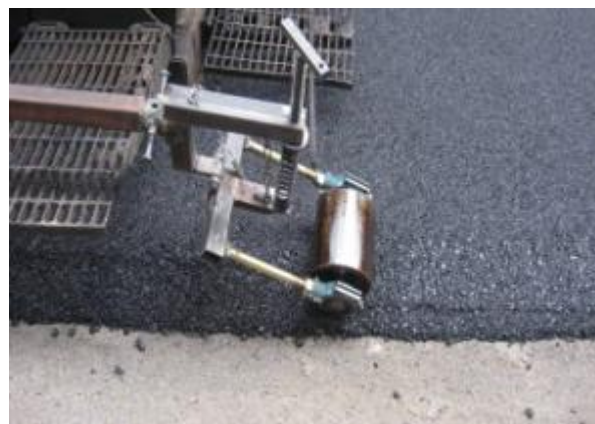
Figure 33. Roller added to compact the vertical edge at the top of the slope.
