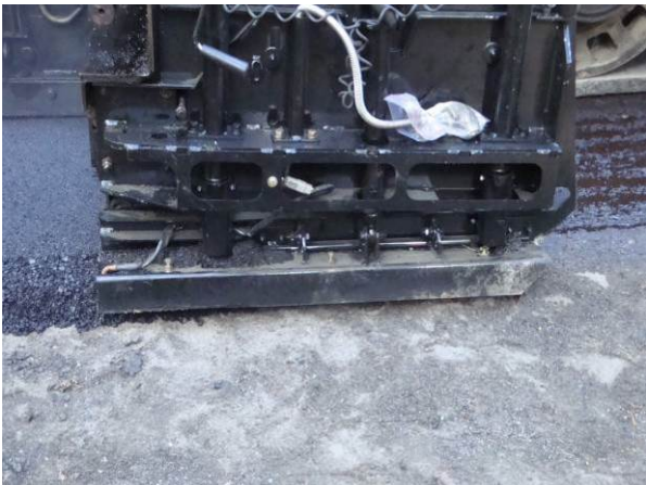
Figure 53. Side view of Carlson end gate.
