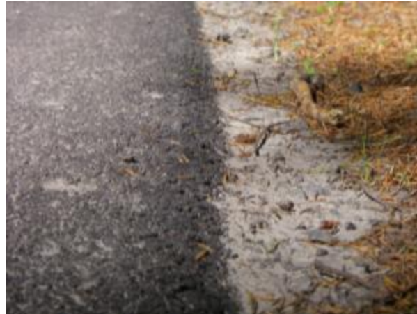
Figure 40. Close-up of pavement edge treatment on SR 410 one year after construction. Shows some exposure of pavement edge treatment.
