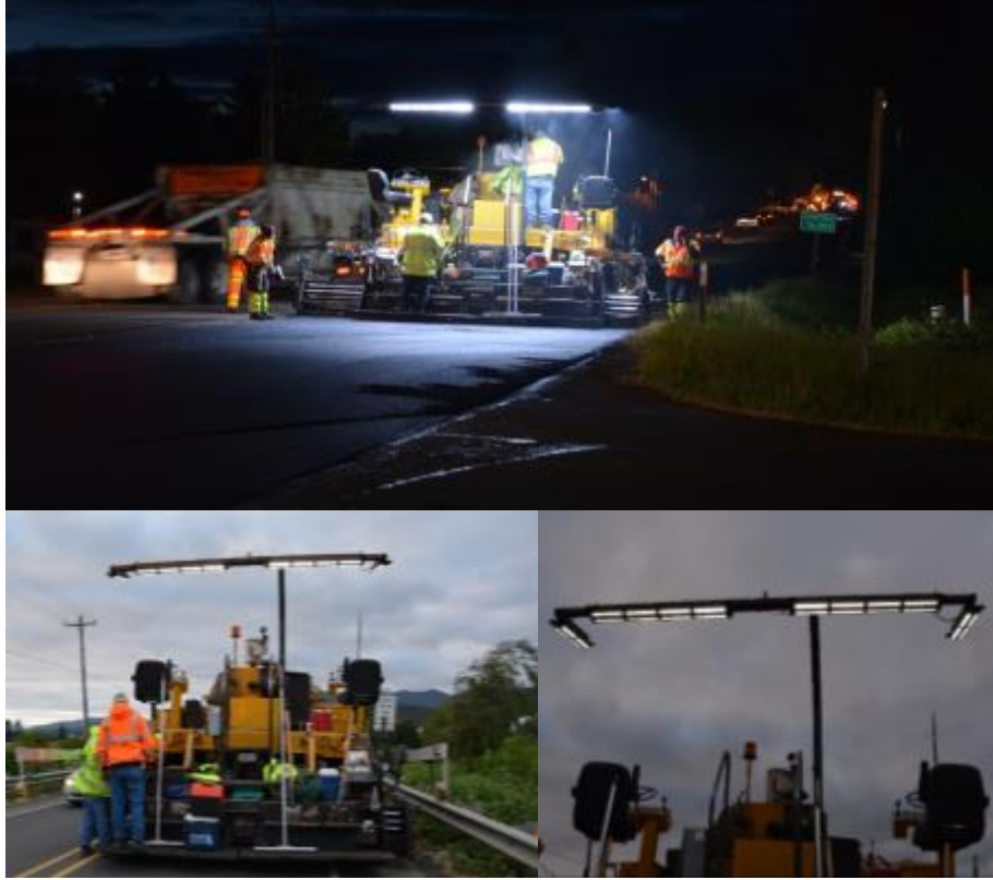
Figure 5.9: Paver with LED Lights
