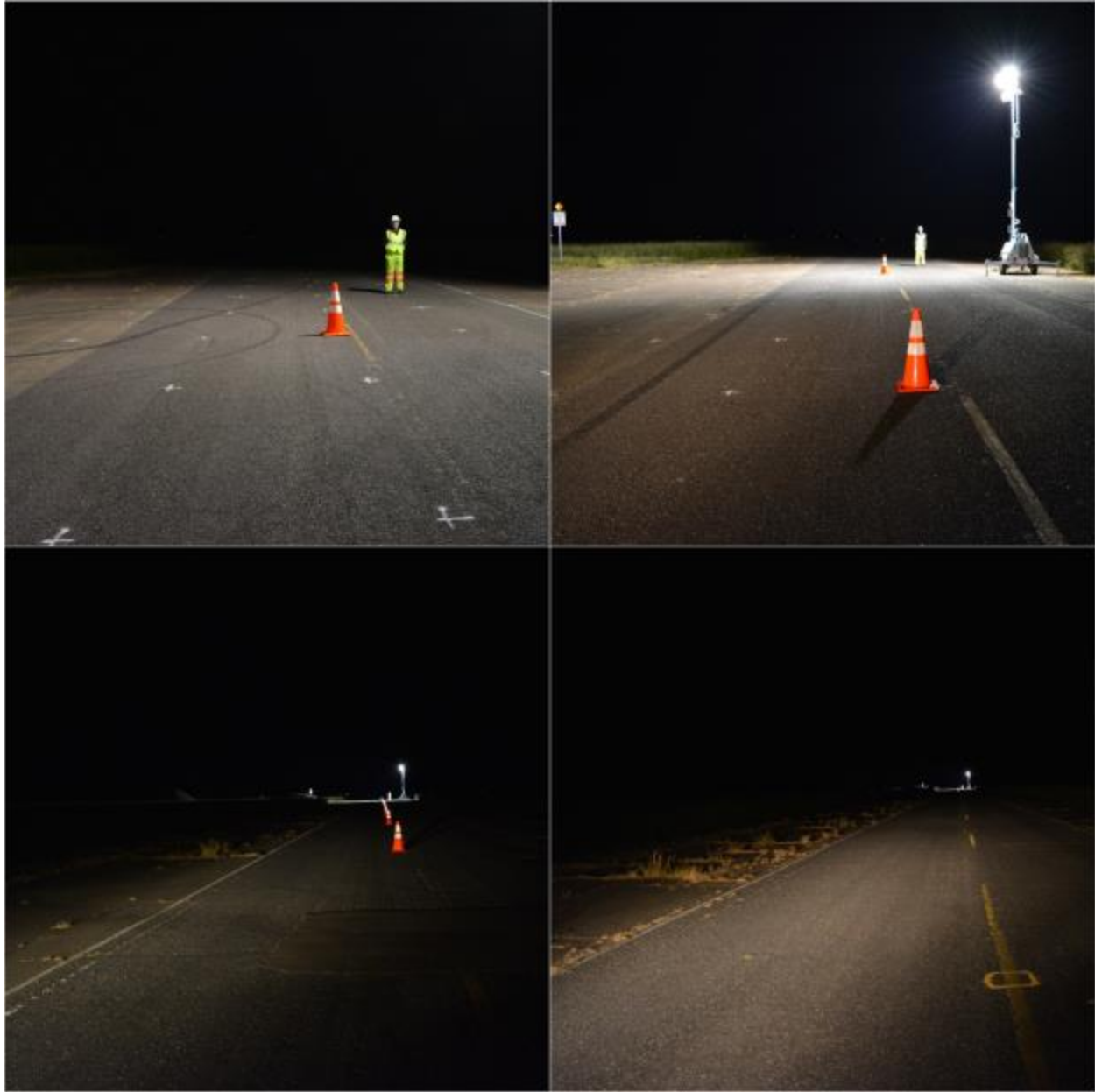
Figure 7.10: Visibility of Worker from Different Distances to Light Tower
