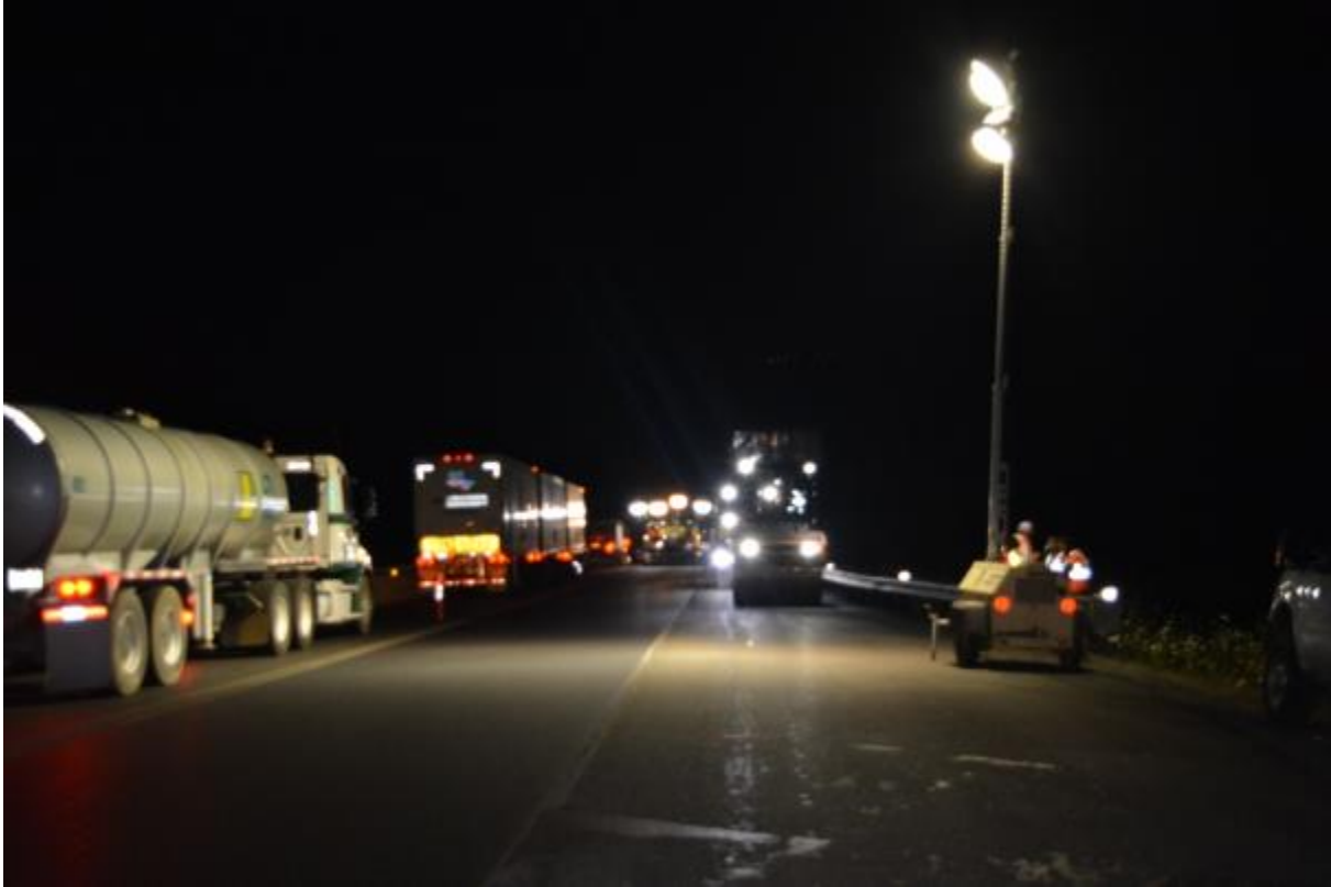
Figure 8.1: Light Tower used on I-84 Jordan Road to Multnomah Falls (Case Study #1)
