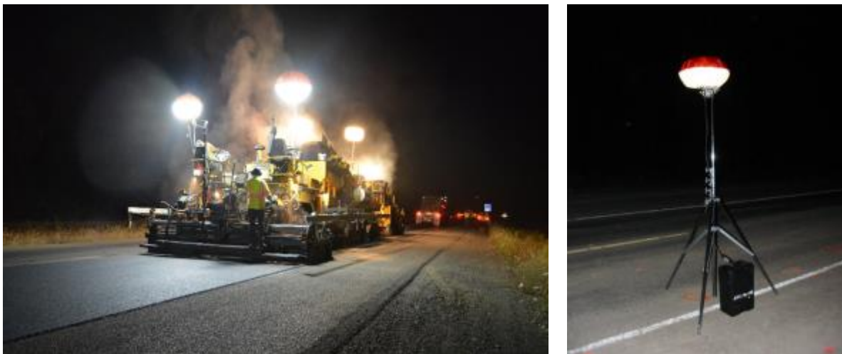
Figure 2.3: Balloon Lights Mounted on Paver (left) and Tripod (right; Gambatese 2005)
