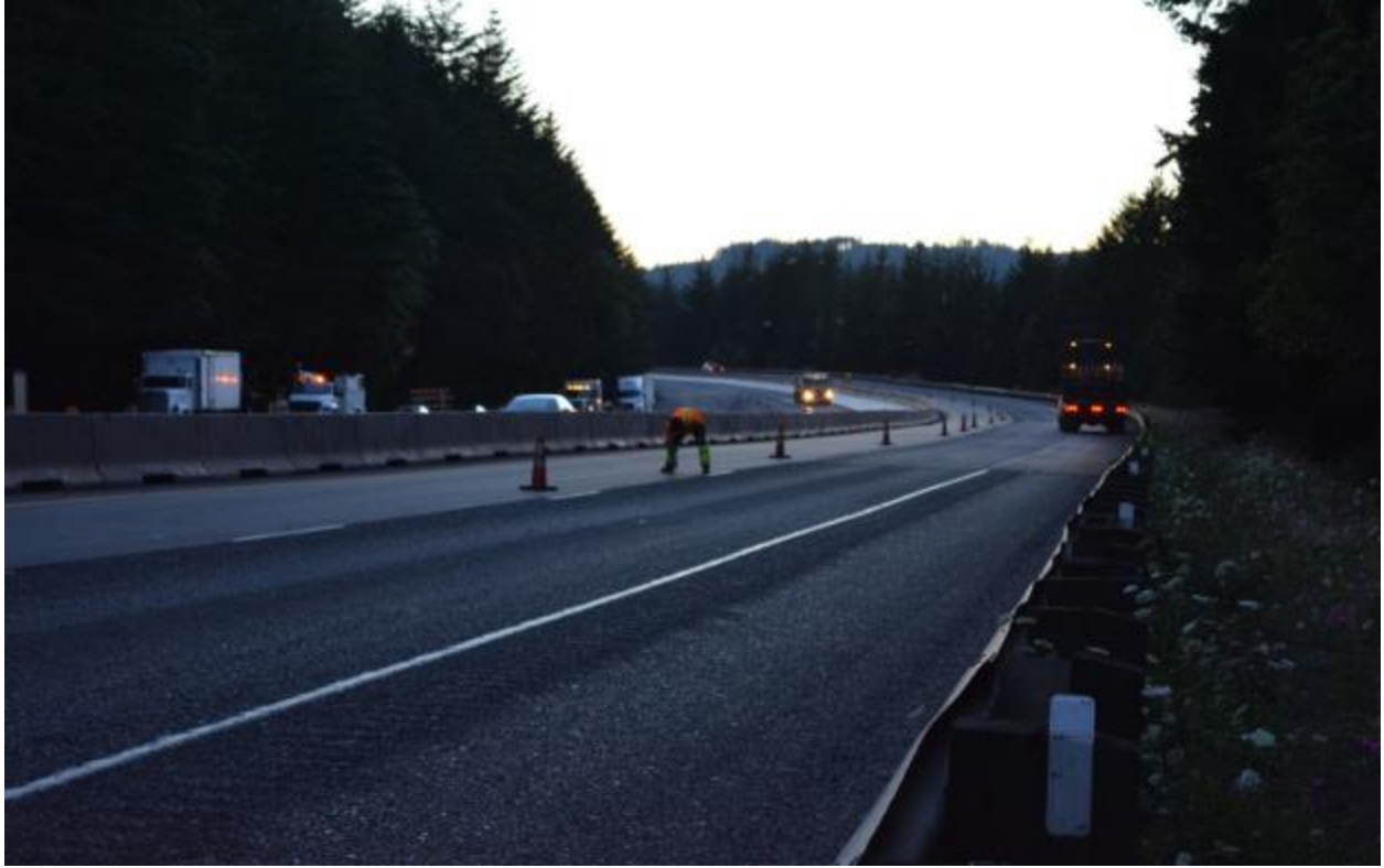
Figure 5.15: Worker in Location without any Temporary or Permanent Lighting
