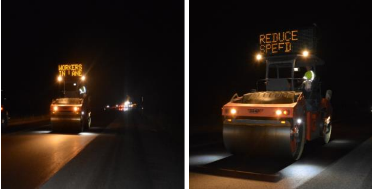
Figure 8.11: Rollers with PCMS Signs, I-84 Jordan Road to Multnomah Falls (Case Study #1)
