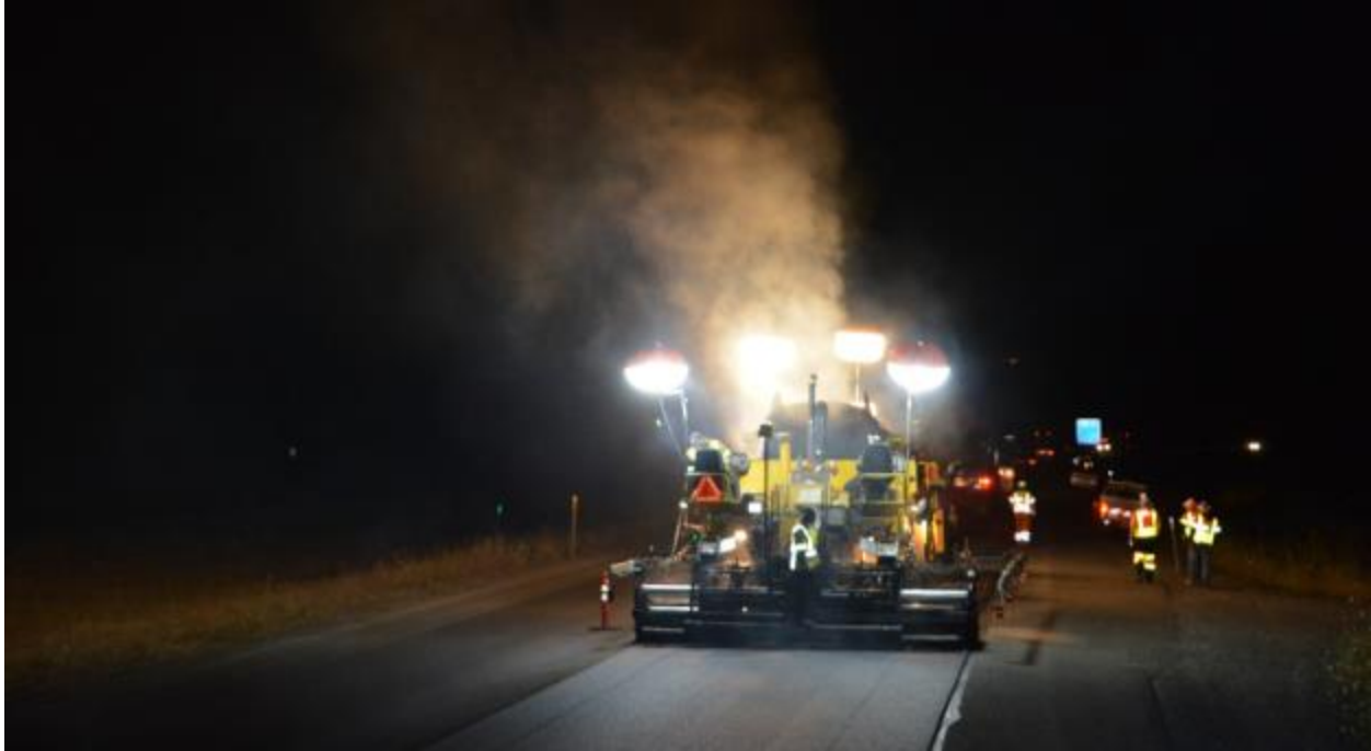
Figure 8.10: Paver with Balloon Lights, I-84 Jordan Road to Multnomah Falls (Case Study #1)
