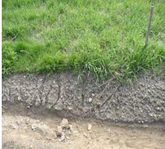
Figure 14. Rill erosion resulting from unprotected ditch slopes (CRWP, 2012)
