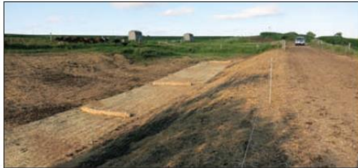
Figure 27. Use of wattle check dams in combination with wood fiber blanket (Brady et al. 2014)
