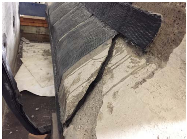
(b) Large cracking above bearing plate
