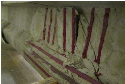
(c) Debonding at epoxy/concrete interface
