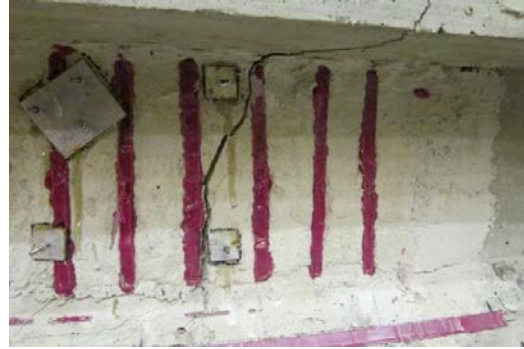
(b) Cracking around CFRP bars in web
