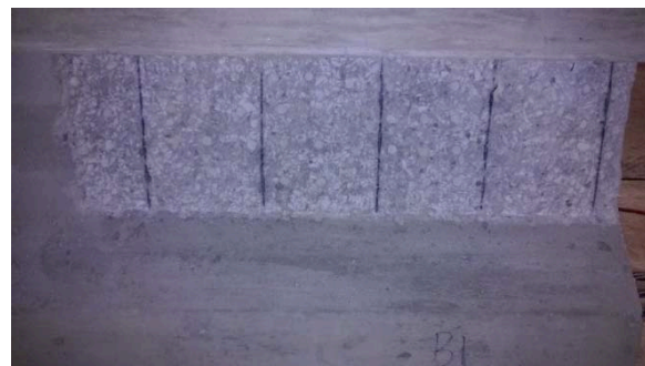
(b) Beam after cover removal
