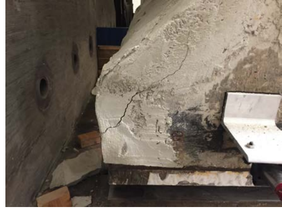
(b) Cracks above bearing plate
