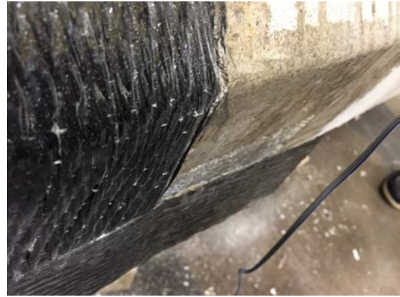
(b) Total debonding of longitudinal strip at ends
