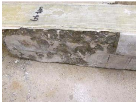
(c) Scaling induced loss of bonded area
