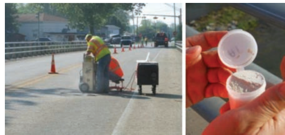
Figure A.4 Chloride ion concentration data collection performed by INDOT (left). Concrete powder sample collected by INDOT (right).
