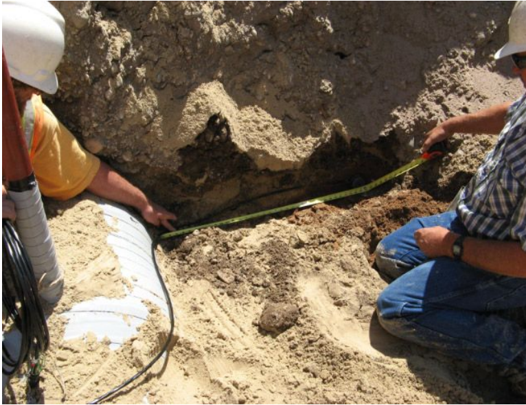
Figure 21 - Placement of the ER probe near the pipe
