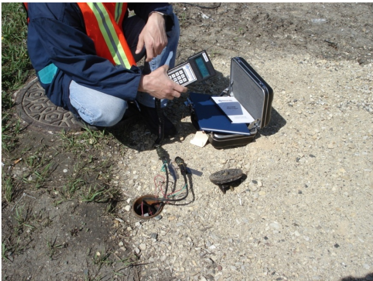
Figure 22 - End terminals at the ground surface for periodic monitoring
