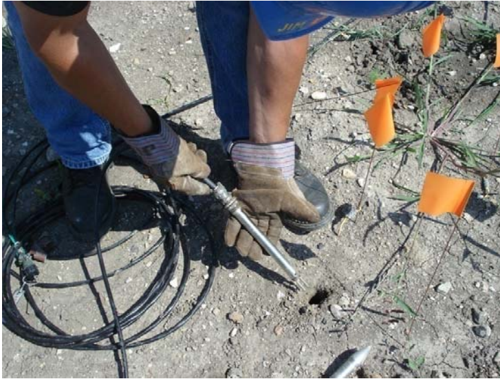
Figure 16 - Installation of the 'Rohrback Cosasco' LPR sensor in test section
