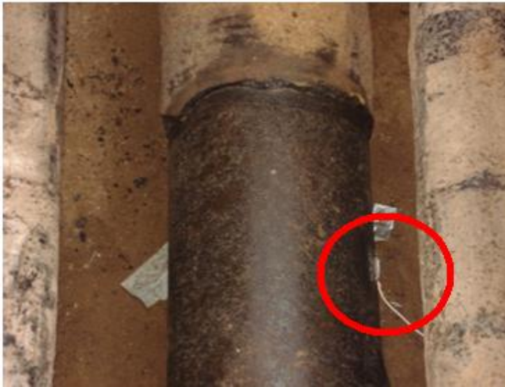
Figure 20 - Welding the ER attached wire to the pipe surface for CP monitoring
