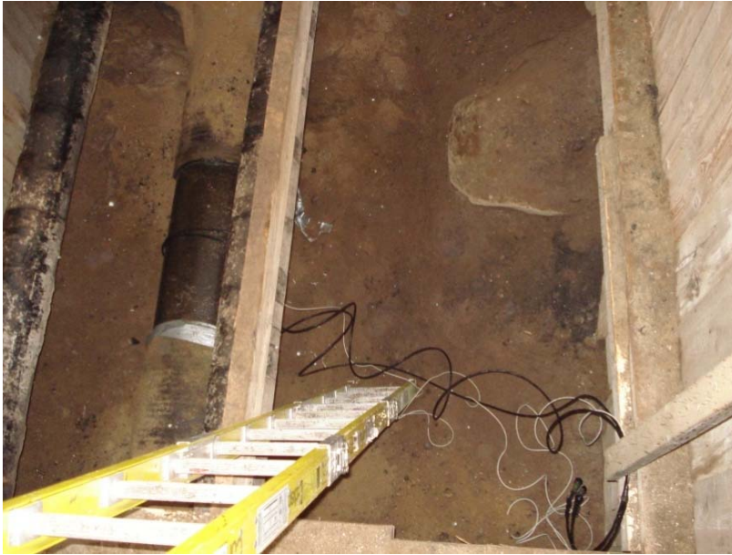
Figure 49 - Installation of the ER probe on the transmission pipe in Utility-A site
