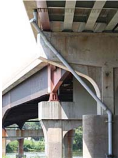
Figure 3. Piping from a bridge deck drain.
