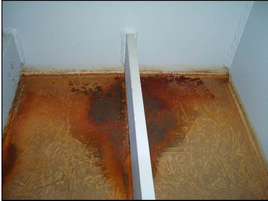
Photograph No. 62 – Looking at the interior of the north cell at the east end of the cap of pier 9. Note: signs of previous standing water on the bottom flange, webs, and stiffeners.
