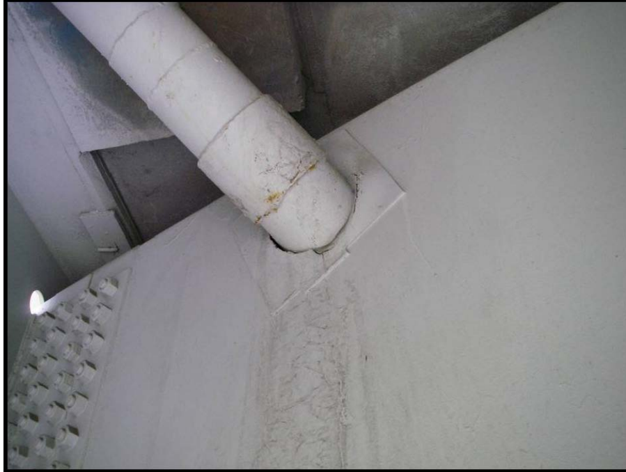
Photograph No. 49 – Looking at the south exterior face of the cap for pier 2A between Girders 4 and 4. Note: the drain pipe is cracked with signs of leakage present.
