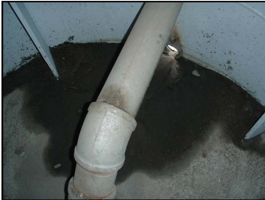
Photograph No. 63 – Looking at the lower drain pipe in the east column of pier 9. Note: the drain pipe is clogged and standing water and wet debris exist on the bottom surface of the east column.
