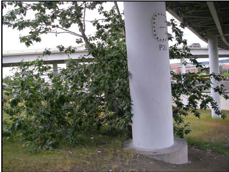
Photograph No. 50 – Looking at the west column for pier 2A. Note: a tree is growing adjacent to the concrete pedestal at the west column.
