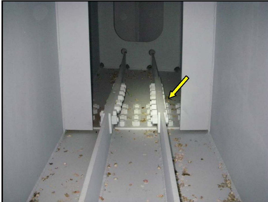
Photograph No. 53 – Looking east inside the cap of pier 4C, in the north cell between Girders 3 and 4. Note: a slight misalignment exists between the bottom flange stiffener
