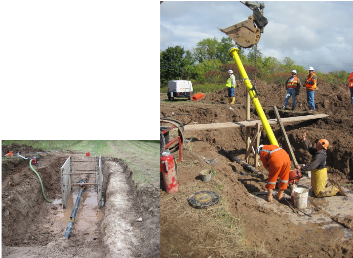
Figure 5.6.4.1: Launching Site B in Oneida, NY; (a) fitting and valve, (b) launcher (yellow pipe) attached to valve.
