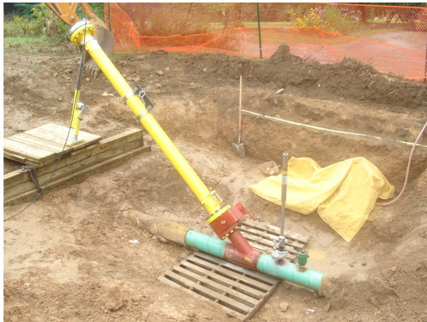
Figure 5.2.4: Launcher attached to pipeline in Brookville, PA
