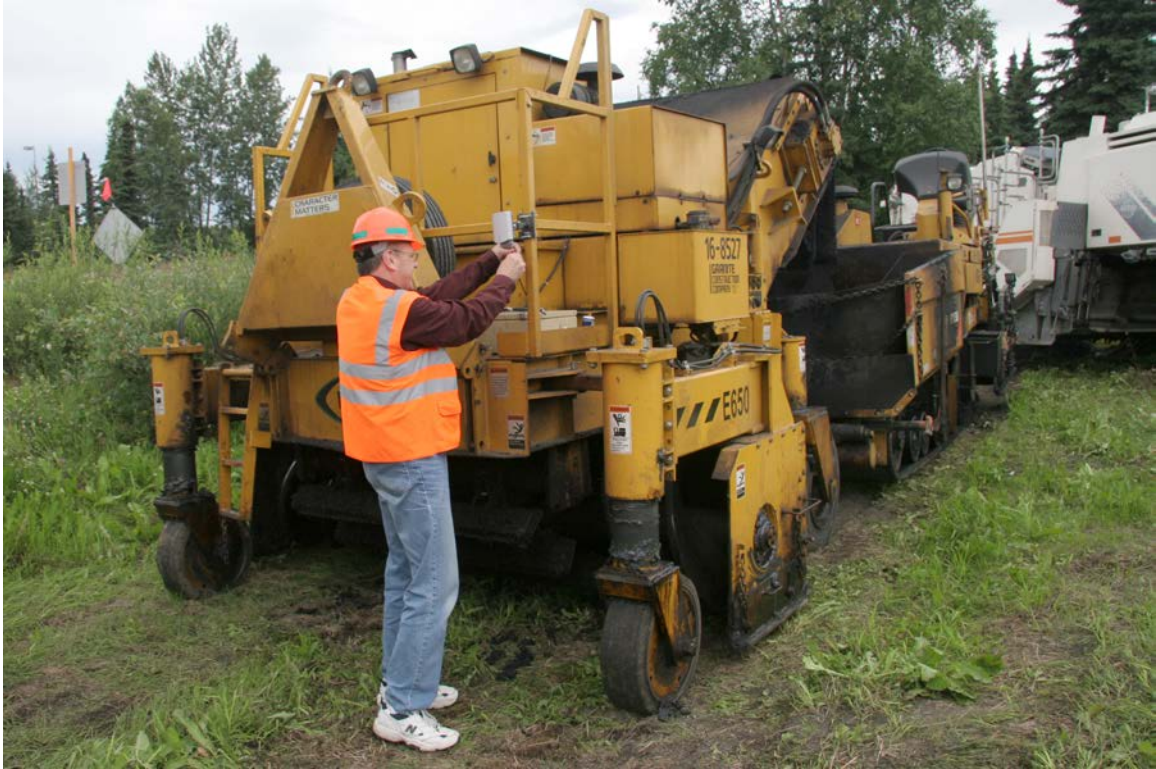
Figure 5.4: Construction paver, CAT AT-1055. Mike Ronchetti is attaching an RF reader. Photo by Janet Burton, University of Alaska.
