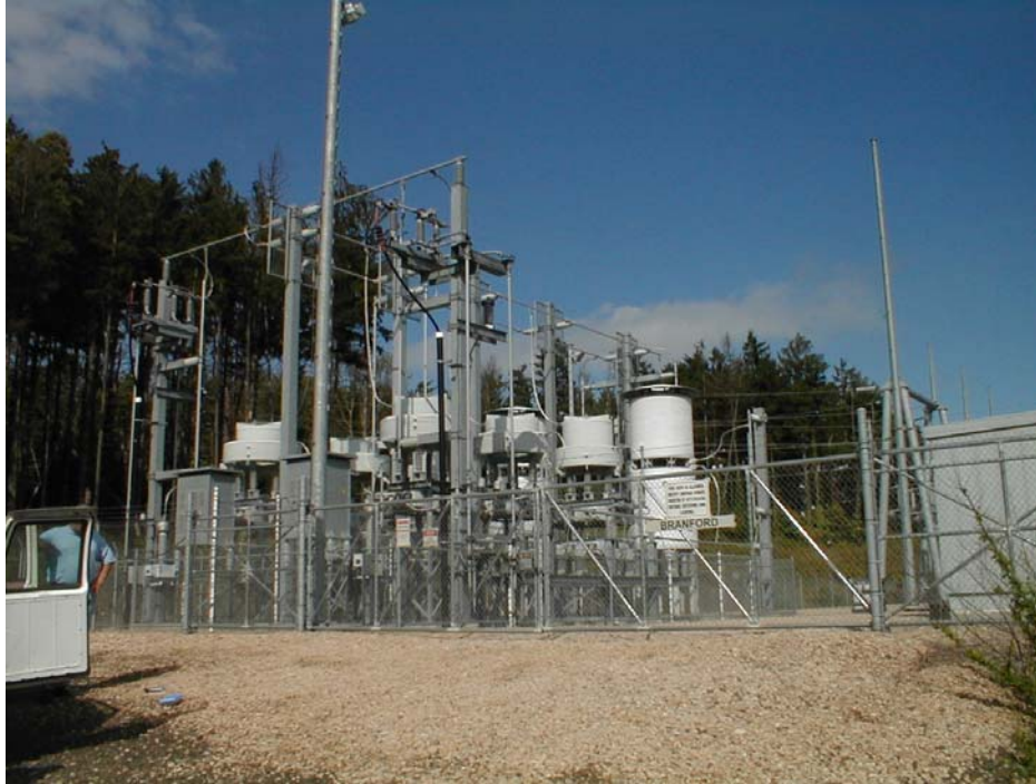
Figure A3. Entrance to Branford SS Showing Filter Bank Equipment
