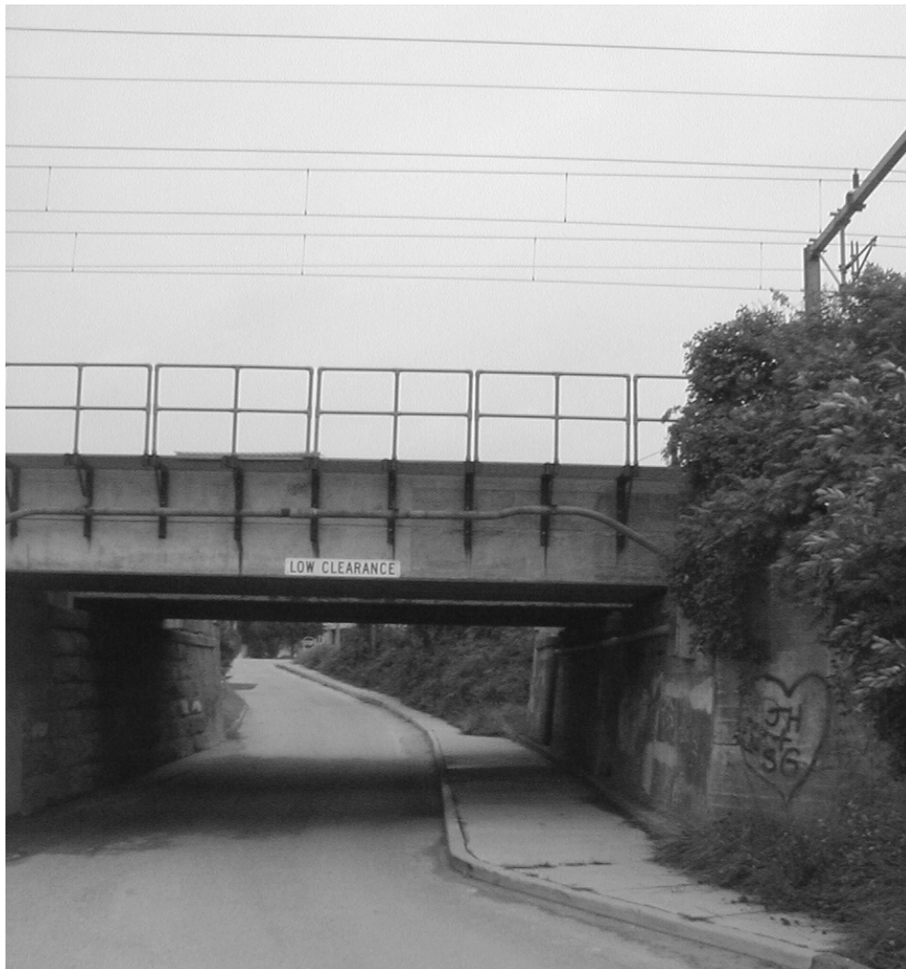
Figure 6. Underpass near the Midway Maintenance Facility. This Road Provides Access to the Bluff Point State Park Situated Beside the Poquonock River
