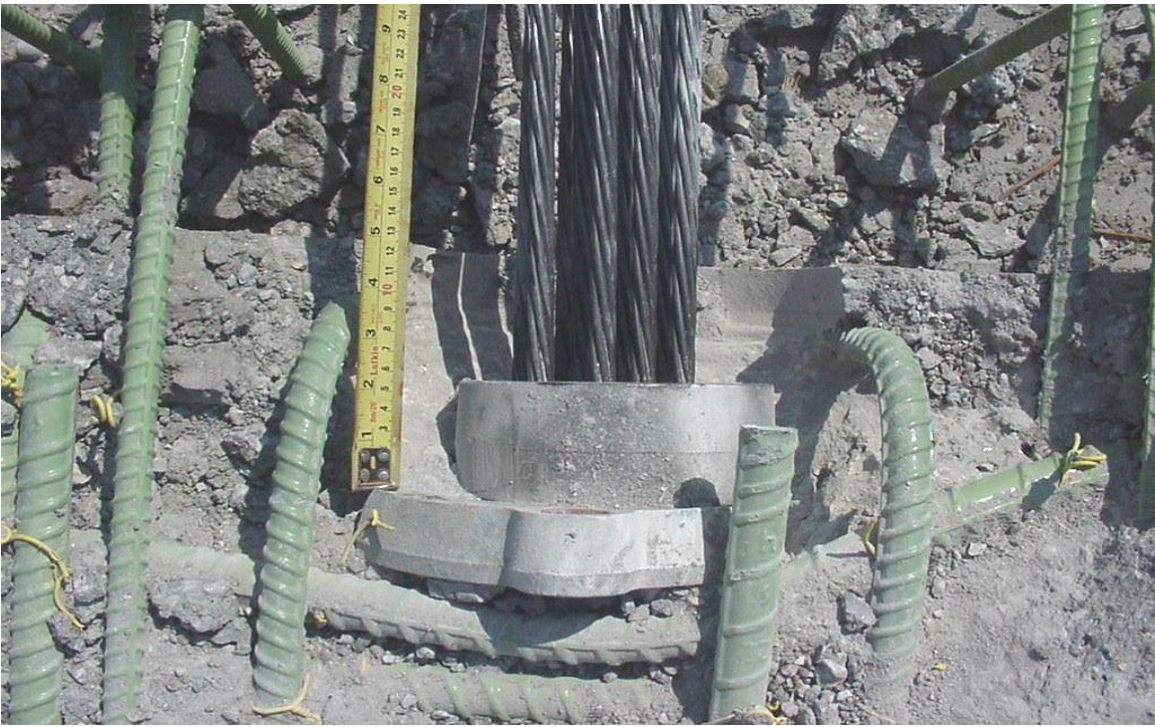
Figure 4. Close-up view of longitudinal anchorage point failure (KDOT).
