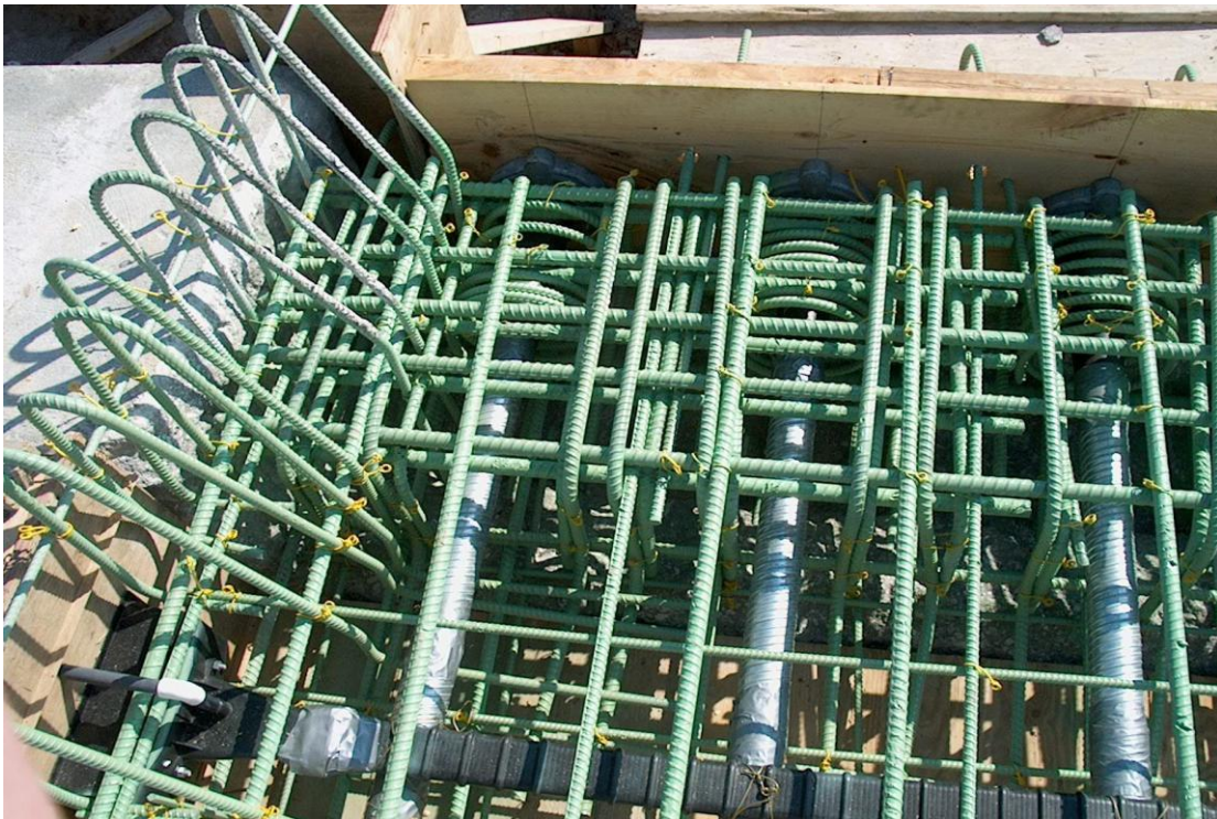
Figure 1. Longitudinal and transverse anchorage points and rebar congestion at bridge abutment (KDOT).
