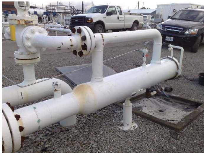
Receive Trap with 2 Bypass Lines
