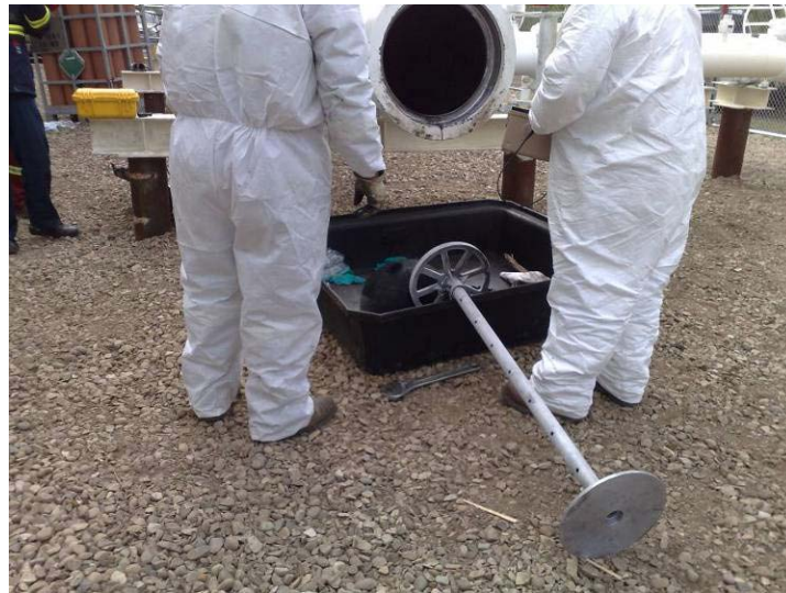
Blocker Bar used in Receive Trap
