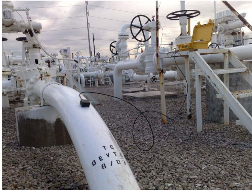
SBR Setup at Receive Trap
