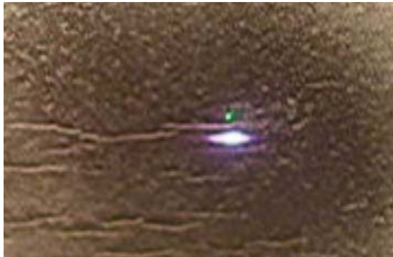
Figure 23 Close-up photo of Crack B shown in Figure 22. This image is the mirror of the one above.
