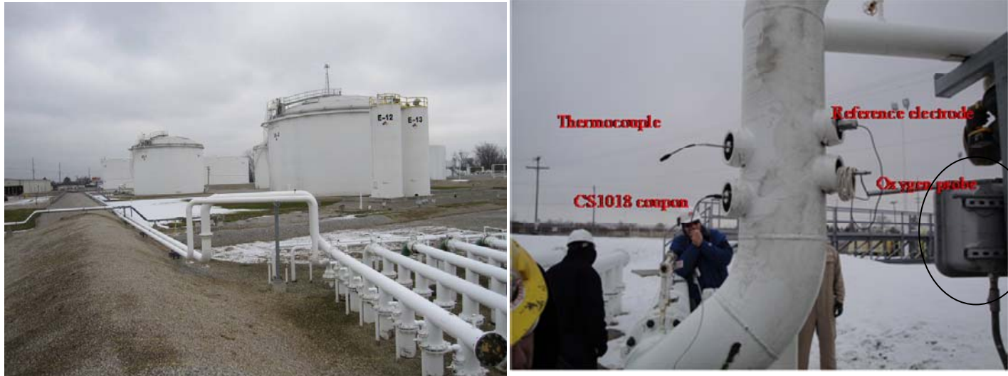
Figure 11. Installation of the probes (right hand figure) at a tank piping in Columbus, Ohio.
