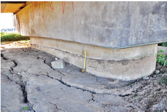
Settlement at Entrance Piers
