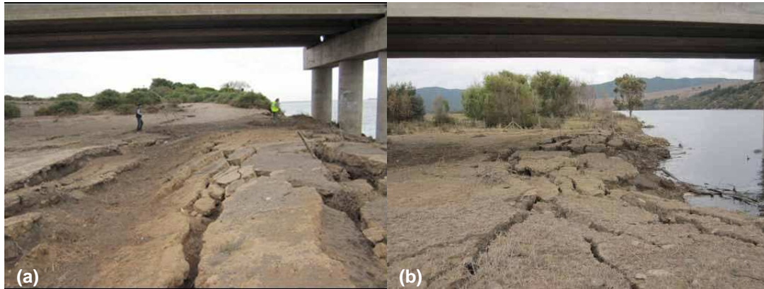
Figure 4.11: Surface manifestation of lateral spreading at Puente Mataquito. (a) Southwest approach (GEER, 2010a). (b) Northeast approach (MAE, 2010).
