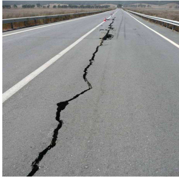
Figure 4.2: Longitudinal crack in northern approach to Puente Mataquito (GEER, 2010a).
