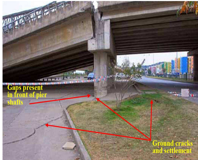
Figure 4.3: Portion of northeast approach to Puente Llacolén affected by liquefaction-induced ground deformation (FHWA, 2011).
