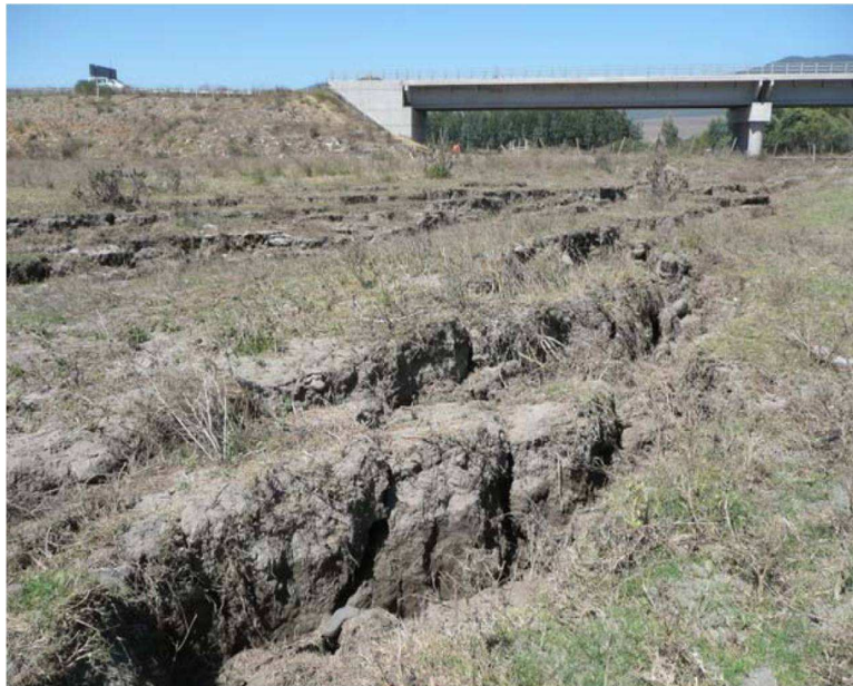
Figure 4.1: Lateral spreading on northern river bank at Puente Mataquito as seen from ground surface (GEER, 2010a).
