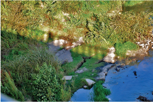
Ground Cracks at the River Bank
