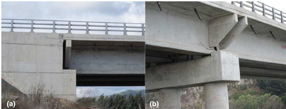
Figure 4.12: Minor structural damage caused by lateral spreading (GEER, 2010a). (a) Crushing of NE abutment. (b) Shearing of bridge girder above interior piers.
