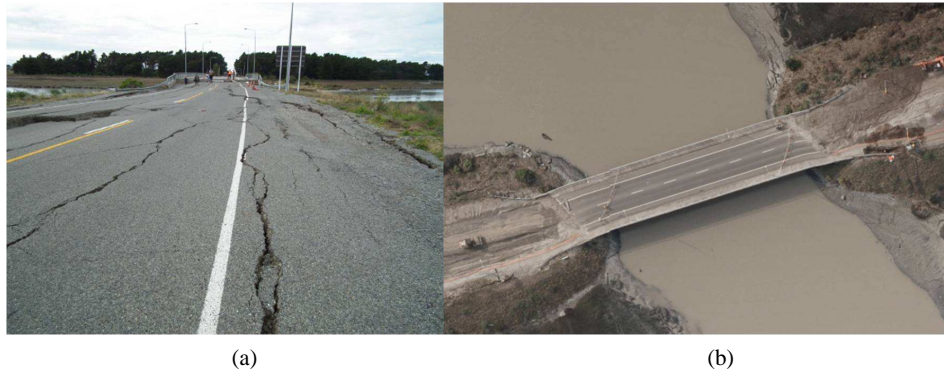
Figure 1.6: South Brighton Bridge after the Christchurch event. (a) Longitudinal lateral spreading cracks in western approach embankment (Cowan, 2011). (b) Aerial photo with visible lateral spreading cracks on river banks (LINZ, 2011).
