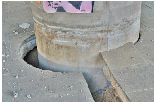
Separation of the Pavement
