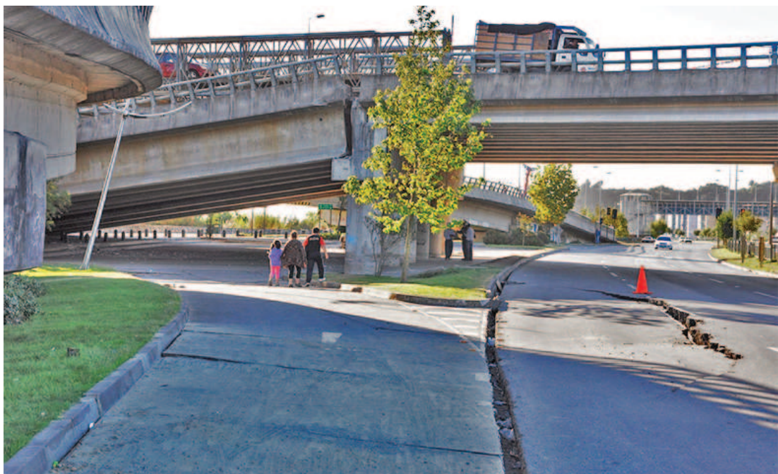
Ground Cracks Extending to the Street
