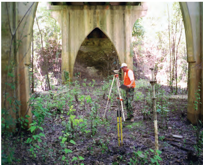
Figure 20. Pier at structure 262050103100 on U.S. Route 501 Business, crossing the Waccamaw River in Horry County, South Carolina (from Benedict, 2003). (Photograph by the U.S. Geological Survey, South Carolina Water Science Center, June 13, 2000).
