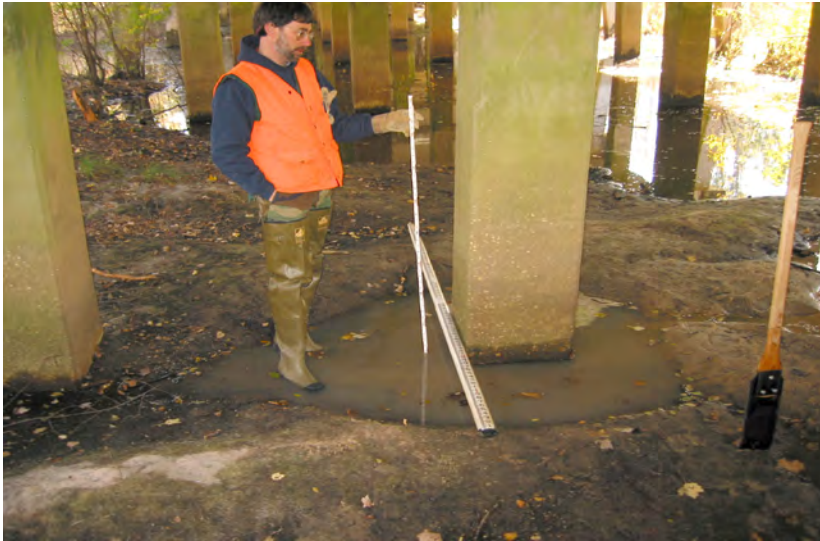
Figure 11. Typical pier-scour hole at structure 342050110800 on U.S. Route 501, crossing the Little Pee Dee River floodplain in Marion County, South Carolina. (Photograph by the U.S. Geological Survey, South Carolina Water Science Center, December 3, 2002)
