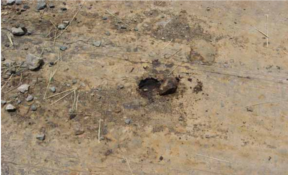
Figure 3.9: Indentation in the Deck Due to Gravel Driven in by the Traffic
