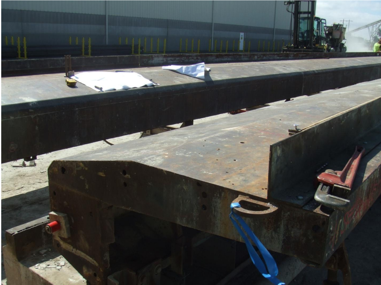
Figure 58. Photo. The bent plate is used to adjust the top flange width of this form. Woodworth 2008
