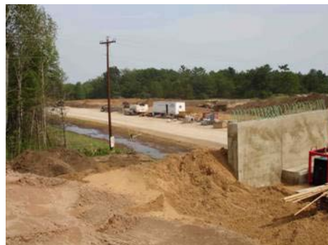
Figure 12. A Segment of Main Line Sub Grade that was Blue Topped because the Model had not yet been Reviewed.
