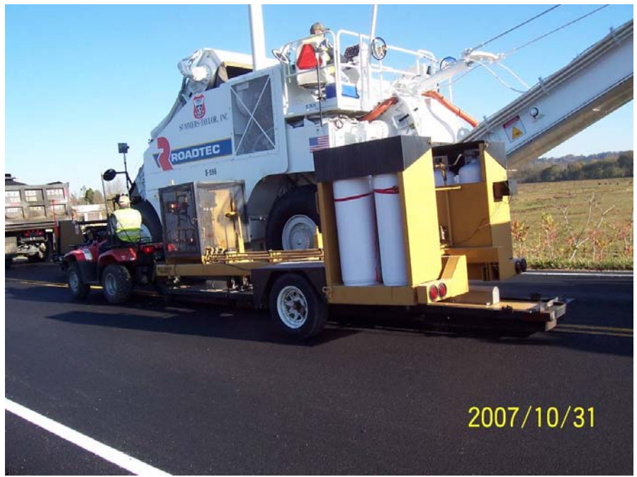
Figure 3-2 Heating Equipment (HDE JM400T)
