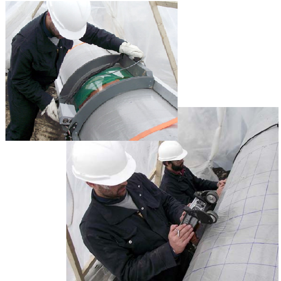
Successful Field Demonstration of MWM-Array Mechanical Damage and Crack Imaging.
