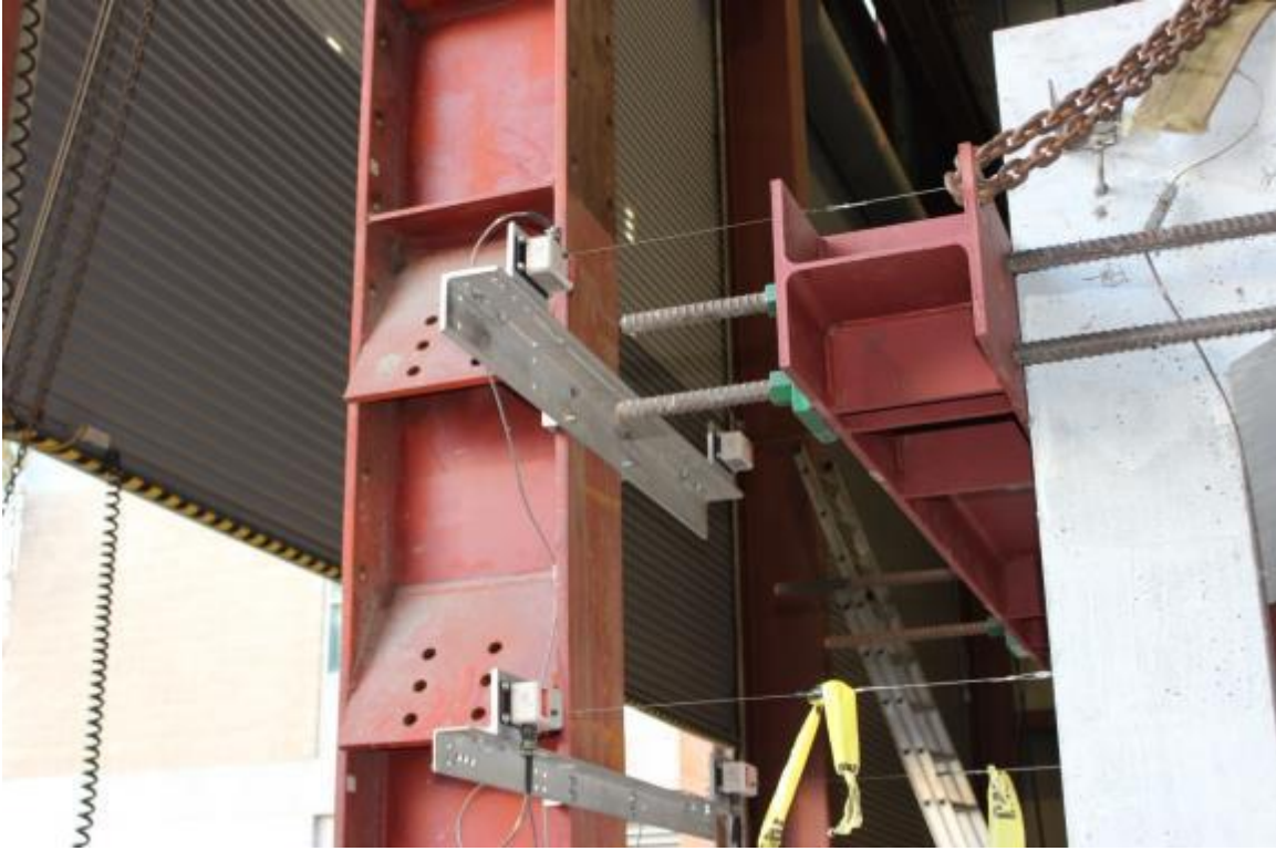
Figure C-14: Installation of loading frame attached to the North wall with 12” long threaded rods
