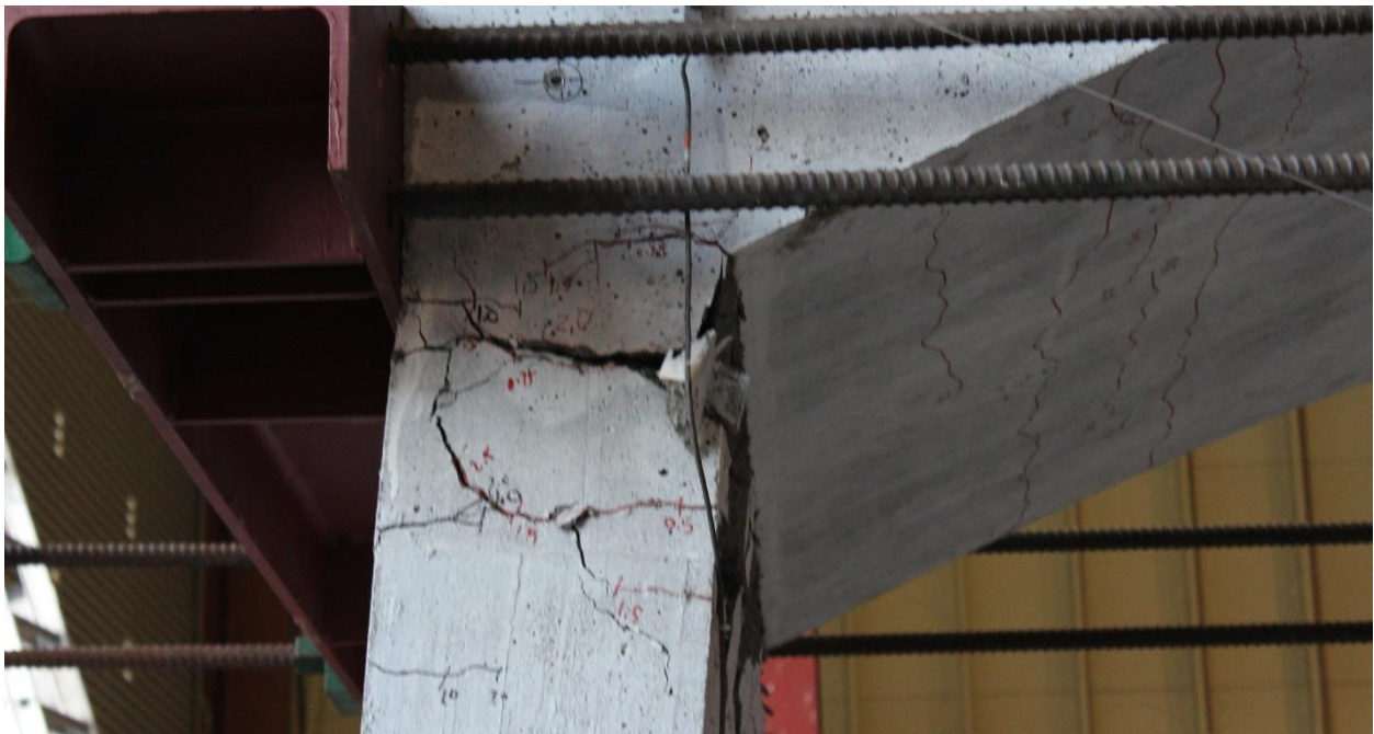
Figure 3-30: North wall roof interface during negative extension at 8.0% drift ratio (Cycle 27-28). Picture of West face at North wall roof interface looking East.
