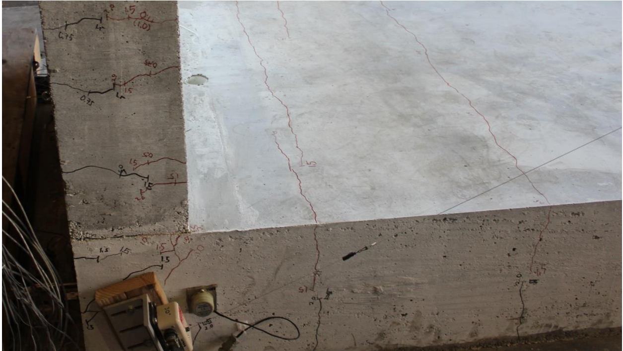
Figure 3-21: Flexural cracks occurring in the base at 2.0% drift ratio (Cycle 11-12). Picture of Southeast corner at base/lab floor intersection looking South-West.
