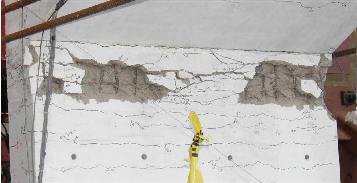
Figure 3-27. Significant concrete spalling at roof/south wall interface during negative extension at 7.0% drift ratio (Cycle 25-26). Picture of inside South wall at roof looking South-West.
