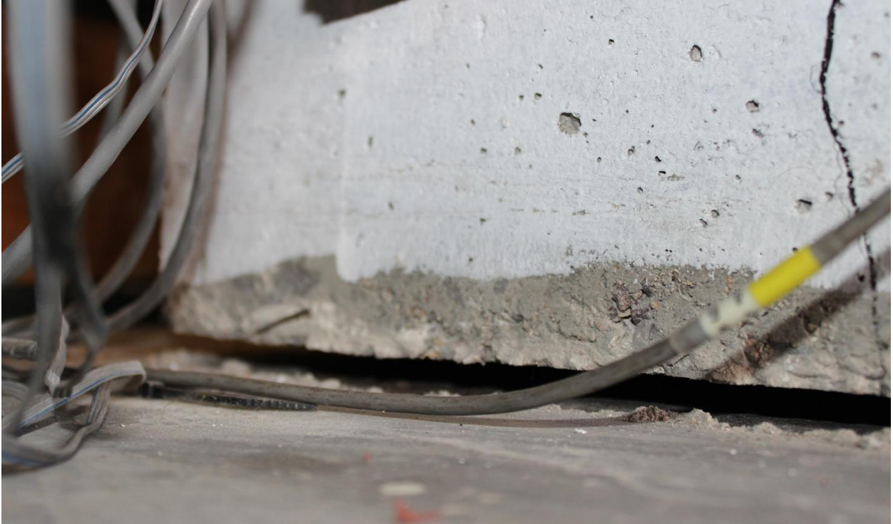
Figure 3-20: Uplift lift occurring at 2.0% drift ratio (Cycle 11-12). Picture of East face at Southeast corner at base/lab floor intersection looking South-West.
