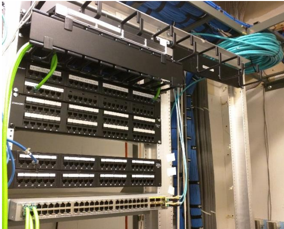
Figure 2.2: Networking equipment in 13 th floor network closet
