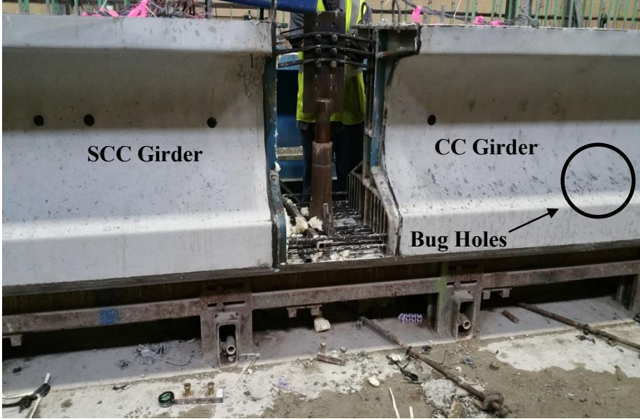
Figure 1-2 Visual side-by-side comparison of SCC and CC girders at the precast plant where both girders have been fabricated through this project
