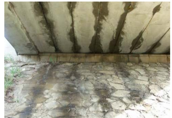
Moisture ingress through cracks and shear keys.
