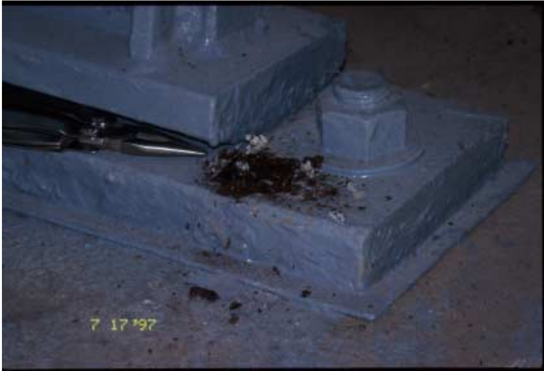
Figure 42. Paint over stratified rust on the bearing.
