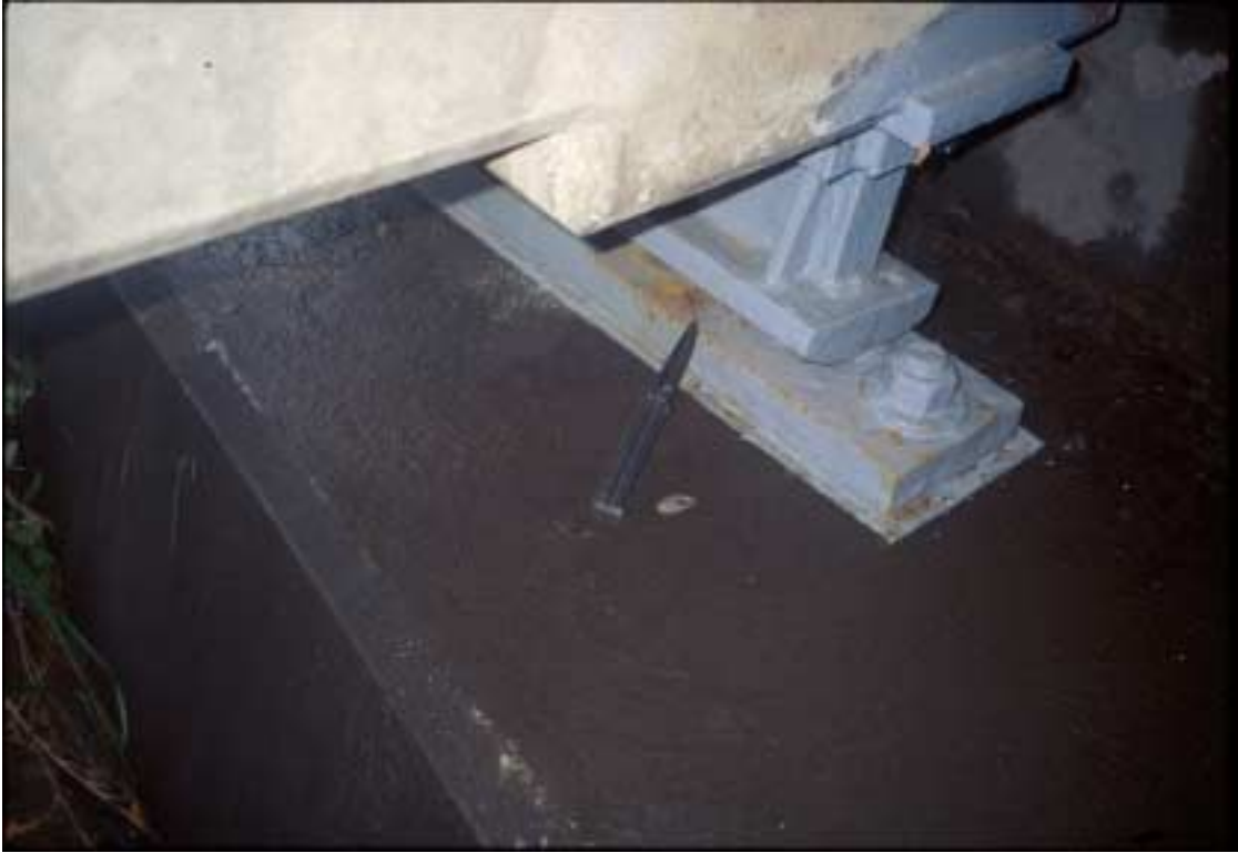
Figure 50. Improper cleaning of the bearing plate.
