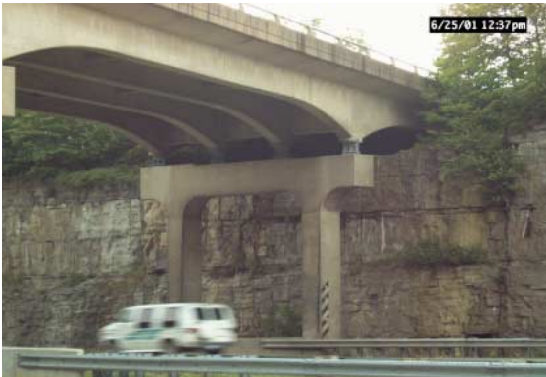
Figure 51. The painted steel rockers of a concrete bridge on an overpass on I-75.
