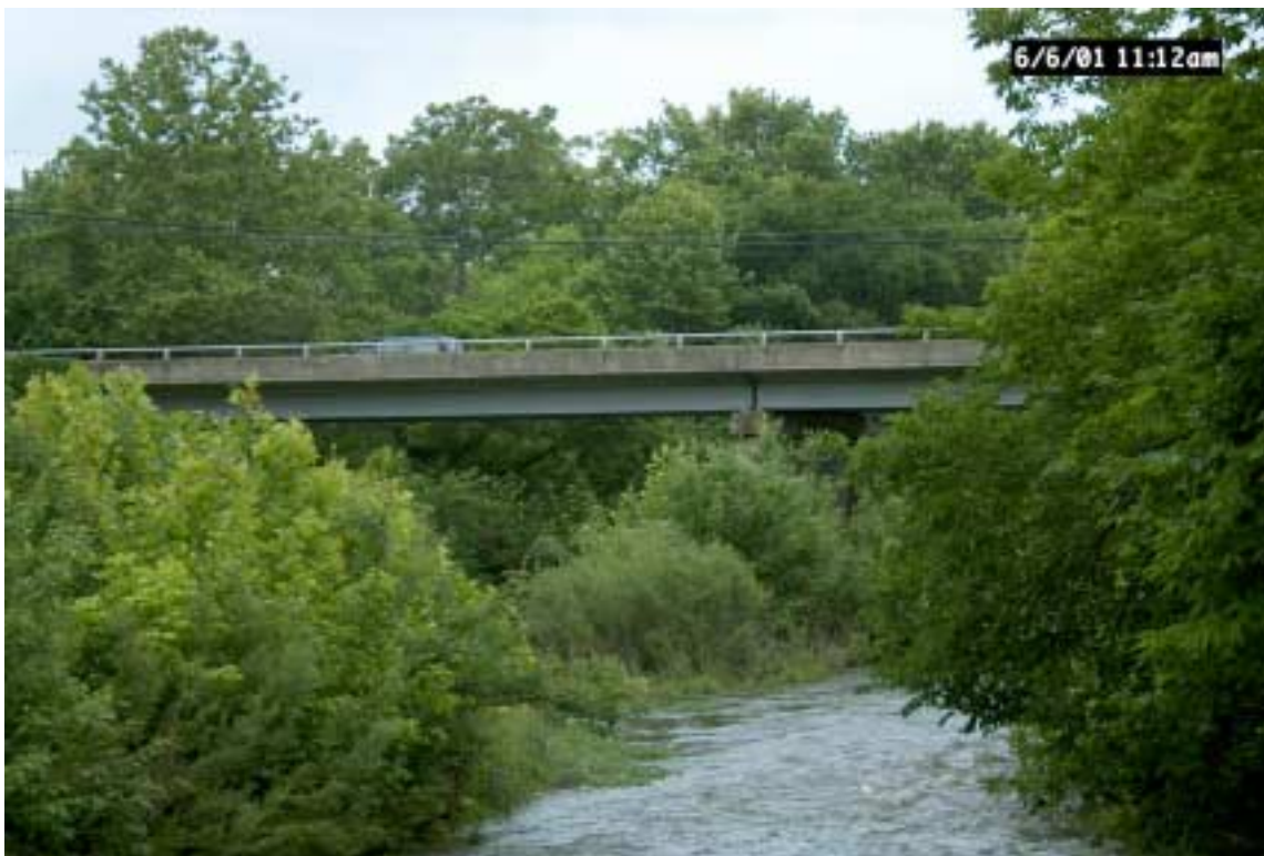
Figure 22. Photo taken during the follow up inspection in 2001.
