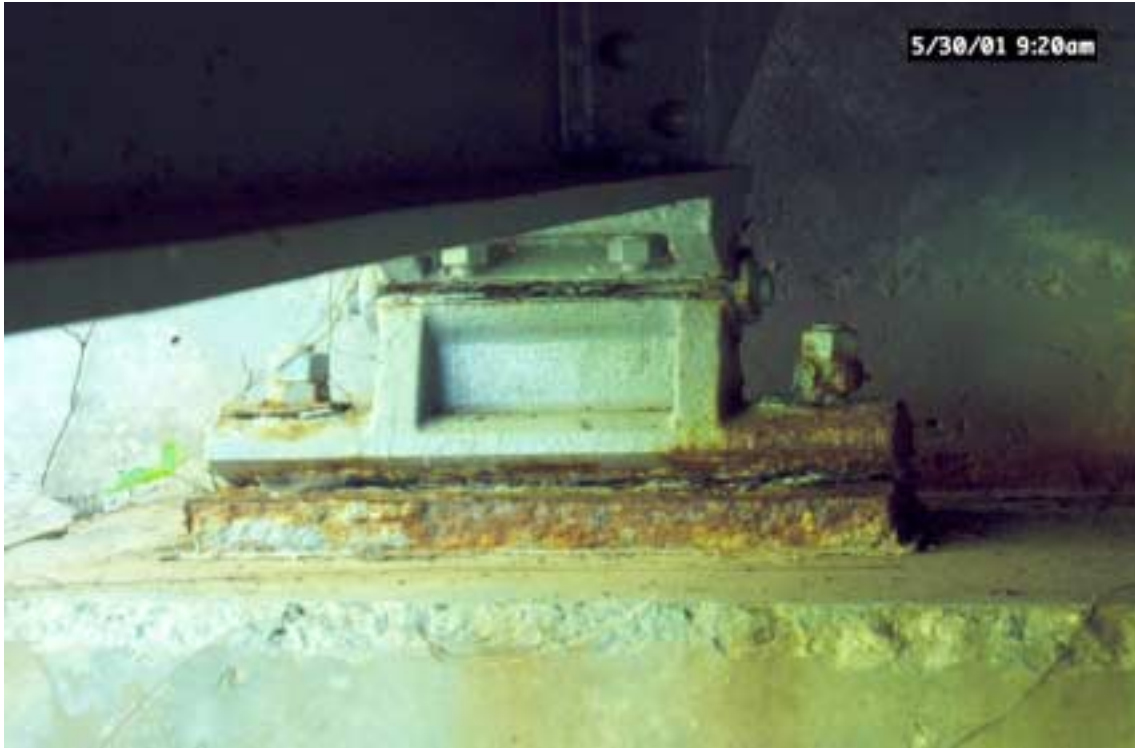
Figure 19. Rust on rocker during follow up inspection in 2001.
