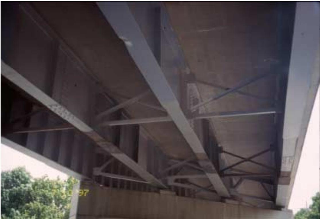
Figure 49. Transition zone of coatings over an overpass on I-75.
