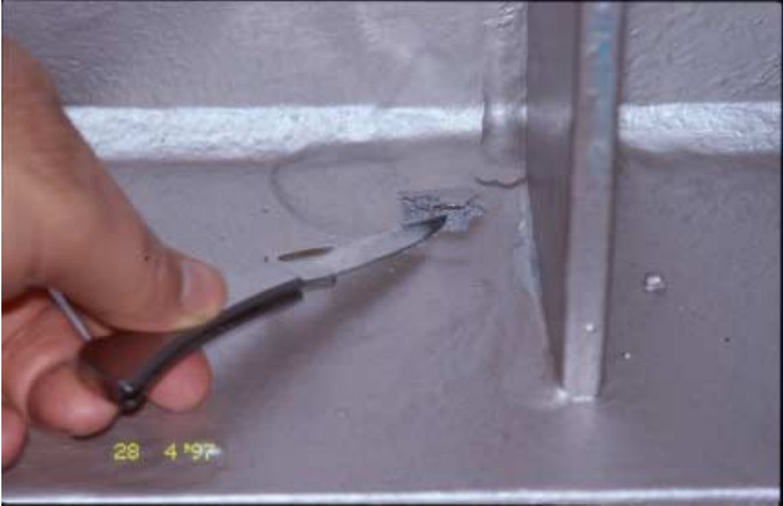
Figure 36. Excessive build up of primer.
