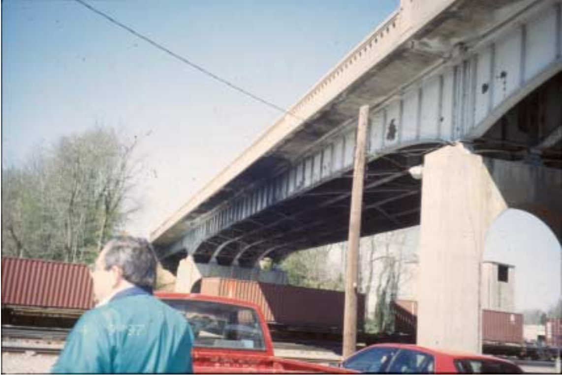
Figure 26. Oil and grease soot on the steel over the railroad tracks in 2001.
