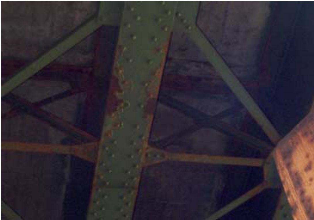
Figure 11. The condition of bridge coating under a construction joint in 2001.
