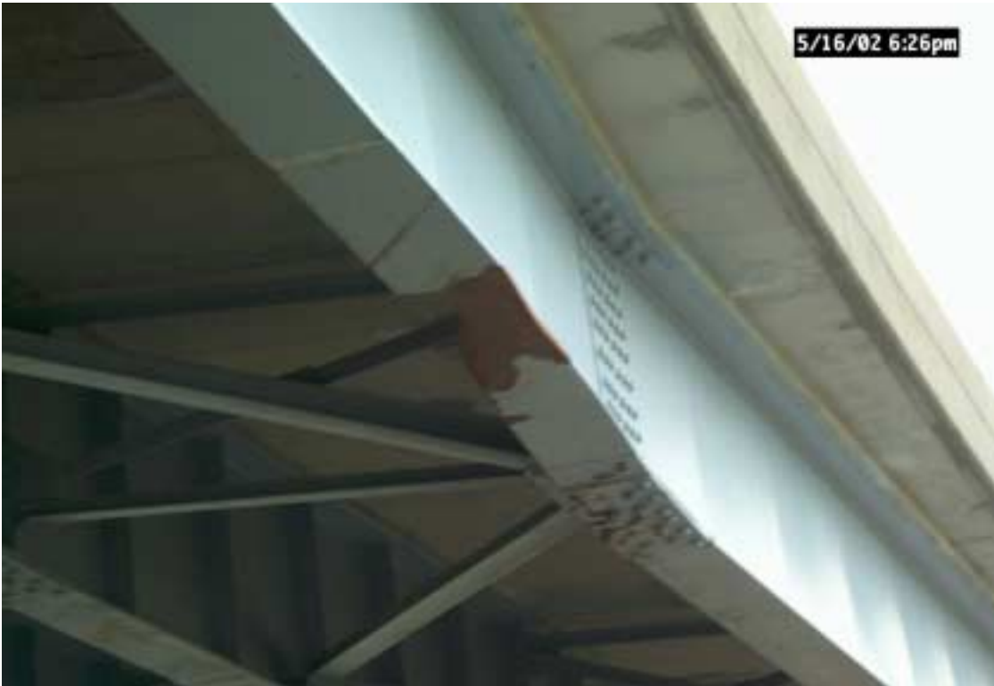
Figure 45. Beam on an overpass bridge damaged due to collision.
