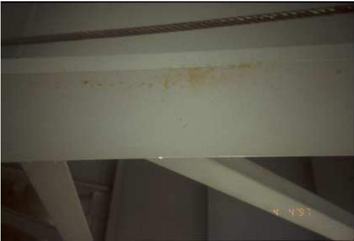
Figure 37. Early rust failure over an overpass bridge on I-64
