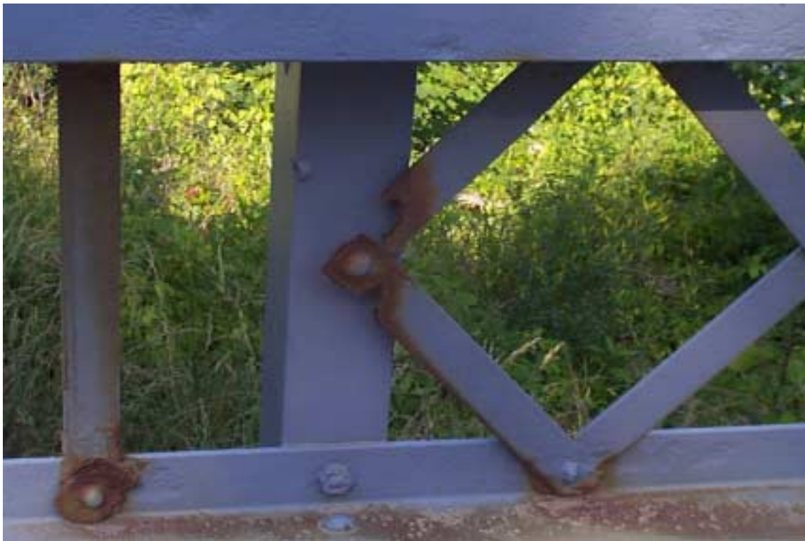
Figure 5. Rusting and separation of welds on the cross bracing.
