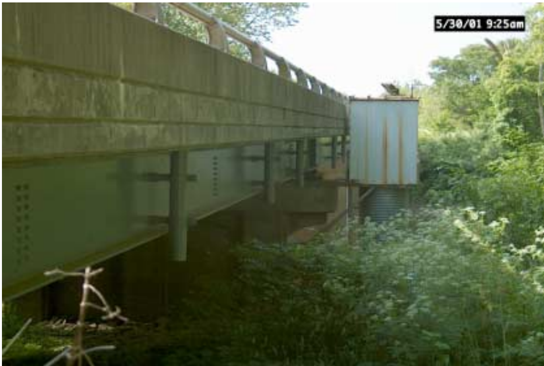
Figure 16. Looking at the KY 55 bridge over Beech Fork River in Nelson County during follow up in 2001.
