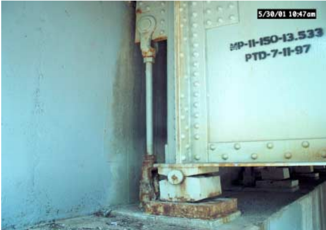
Figure 28. Condition of the rocker in 2001.
