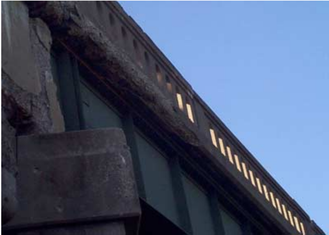
Figure 12. Deteriorated concrete on the abutment.
