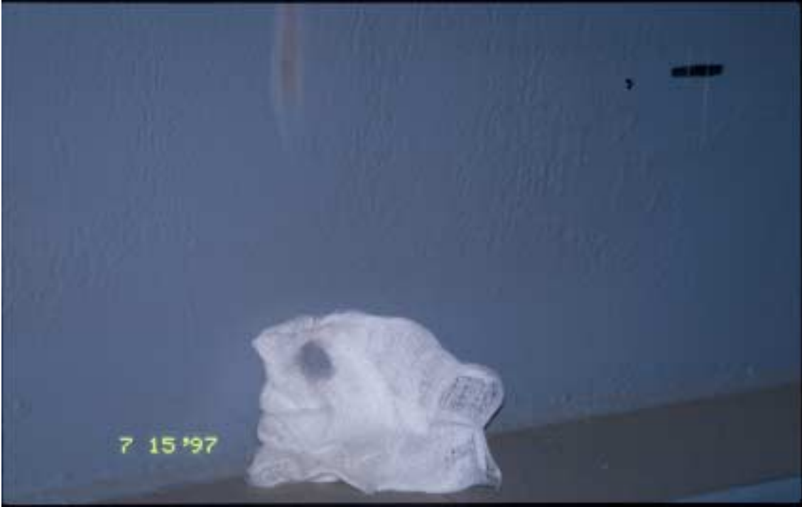
Figure 38. Improperly mixed top coat.
