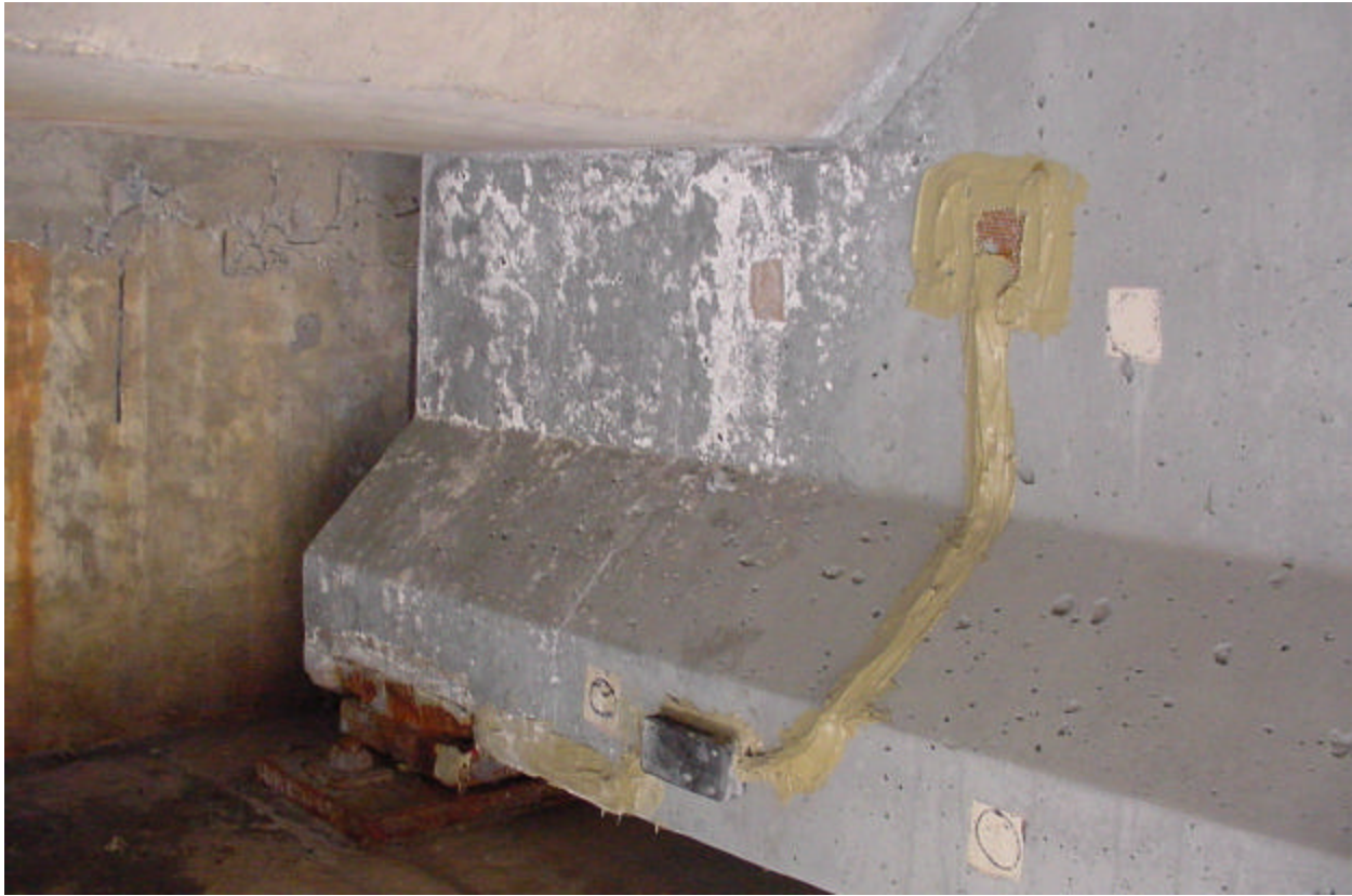
Photo 7. Beam 2 west side Zn/Al anode corrosion products.
