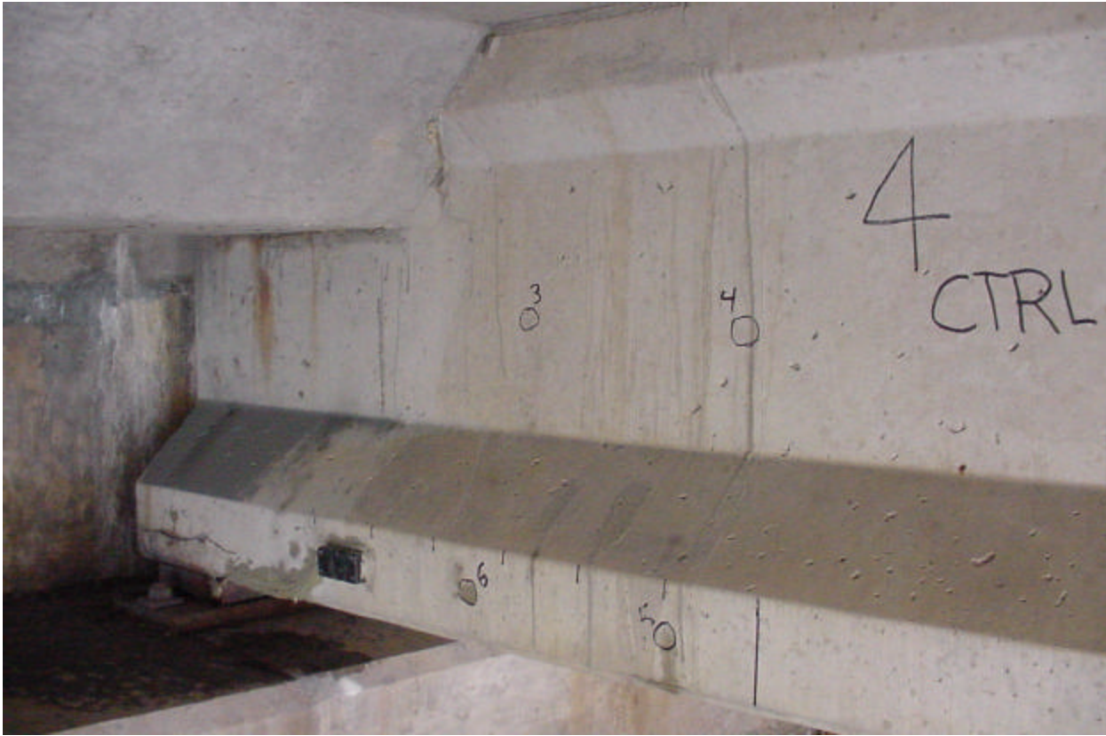
Photo 8. West side of Beam 4. Little evidence of water running down the face of the beam.
