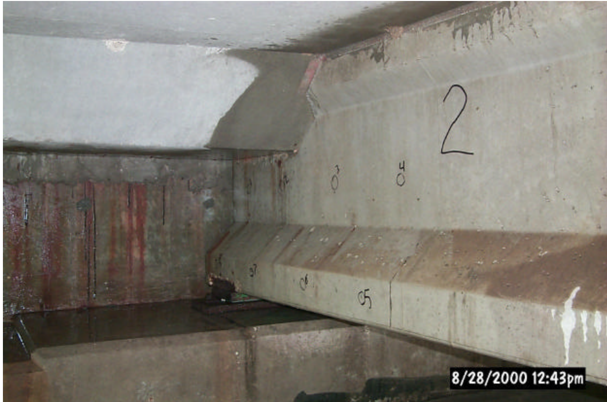
Photo 1. Power washed beam #6 with corrosion potential sites located. Note test locations detailed by numbered circles.
