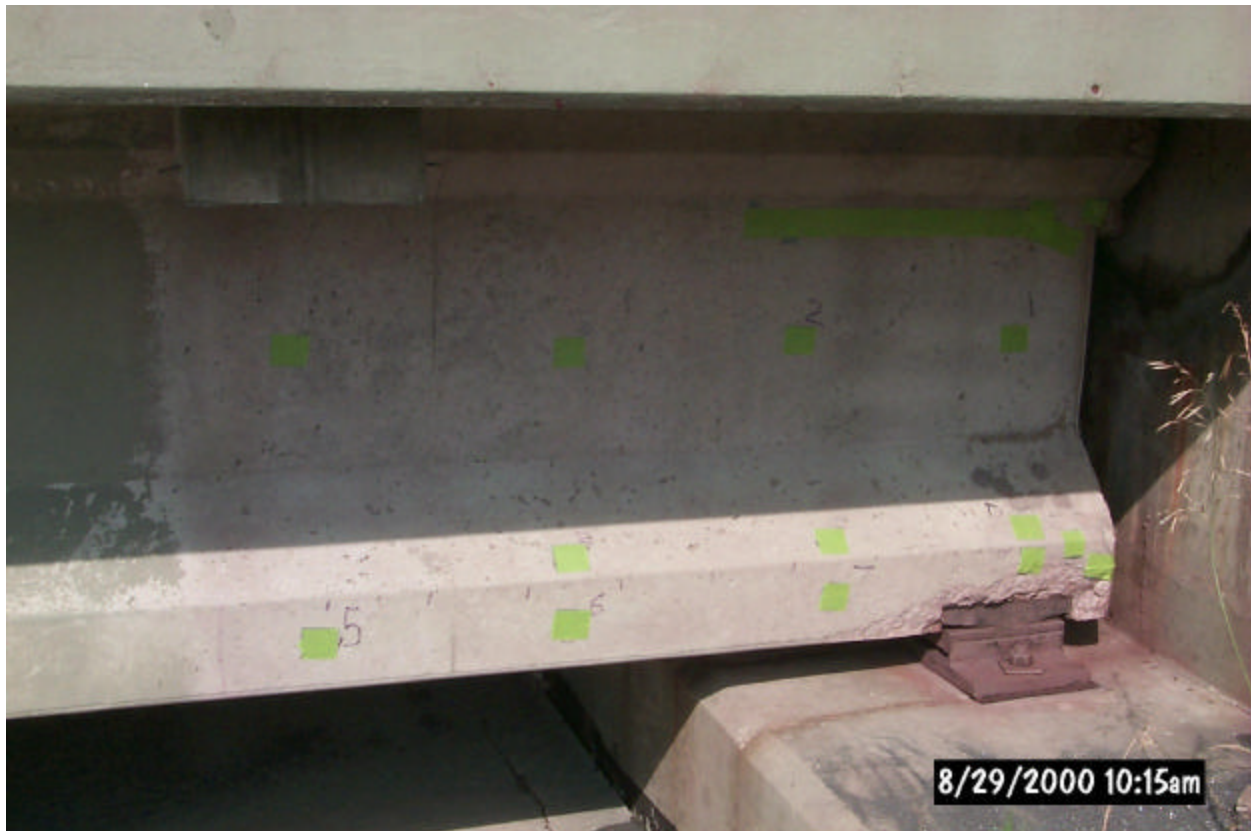
Photo 3. Beam #6, east side w/fiber tape cover over corrosion potential sites and exposed metal tie wires.
