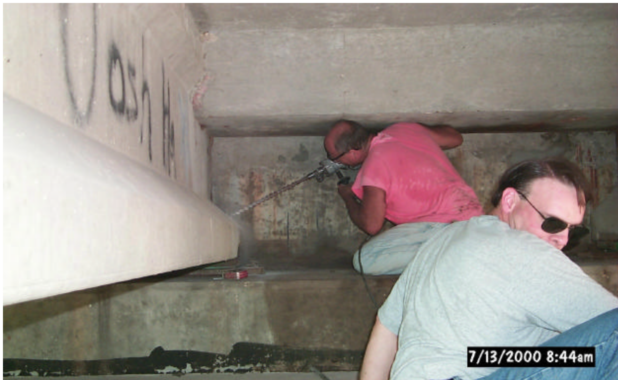
Photo 2. Removing concrete cover from stirrup.
