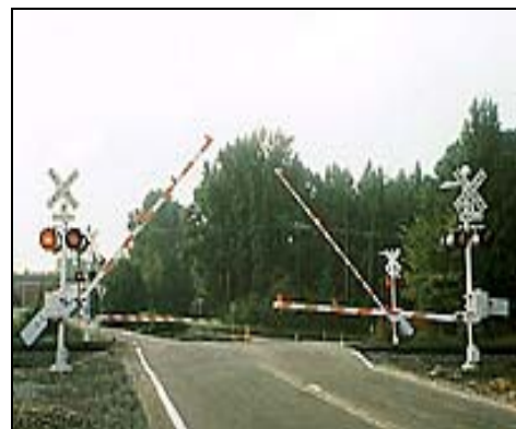
Figure 5. 4-Quad Gates at West Craighead Road, Charlotte, NC
