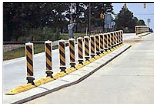
Figure 7. Traffic Channelization Device at Hickory Ridge Road, Harrisburg, NC
