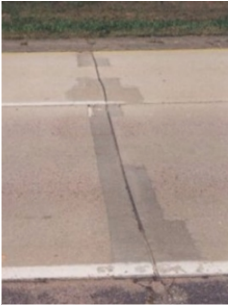
Figure 3 Joint 685 before minimum rehabilitation.
