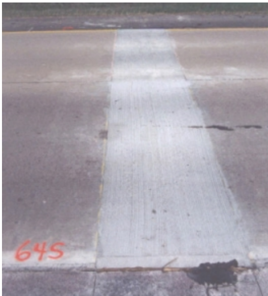
Figure 16 Joint 645 contains Strata Grid-200, with maximum rehabilitation and an unsawed joint prior to the asphalt overlay.
