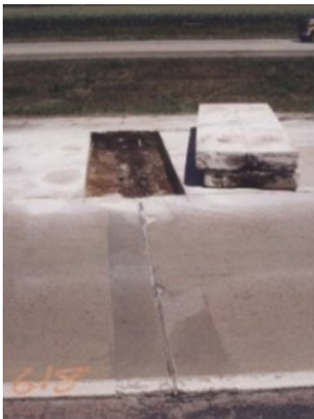
Figure 1 Joint 618 following the removing of the four-foot section and prior to the insertion of the steel bars and concrete.
