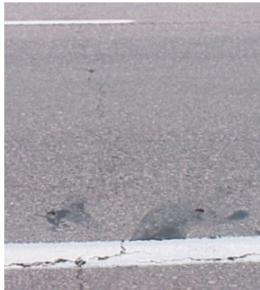
Figure 17 Joint 645 with crack reflecting through the asphalt overlay where the joint is.
