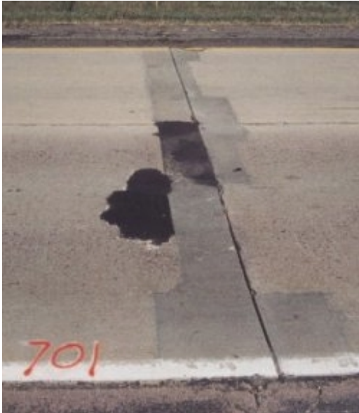
Figure 18 Joint 701 with no fabric, an unsawed joint, and minimum rehabilitation prior to the asphalt overlay.
