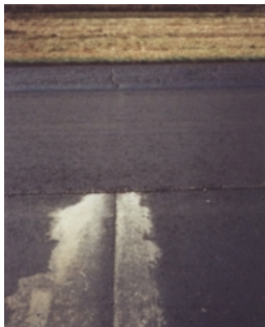
Figure 14 Joint sawed after asphalt overlay.
