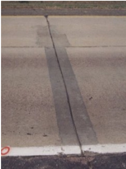
Figure 20 Joint 730 with no fabric, minimum rehabilitation, and a sawed joint prior to the asphalt overlay. (note the partial depth repair that was completed in 1979)
