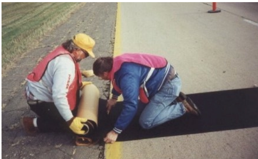
Figure 5 Supplier-Personnel and Gill Hedman (Office of Materials and Surfacing) installing Linq Tac-711N.
