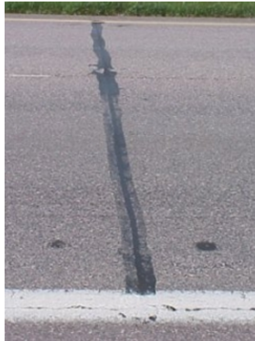
Figure 21 Joint 730 showing no problems with the joint. (More typical performance of minimum rehabilitation)
