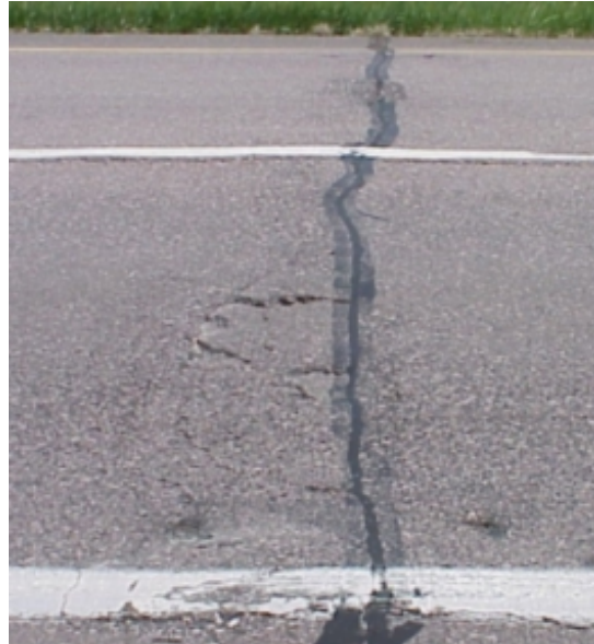
Figure 19 Joint 701 with buckling of the concrete causing cracks to reflect through the asphalt overlay. (Only minimum rehabilitation joint that showed buckling problems in the entire test section.)
