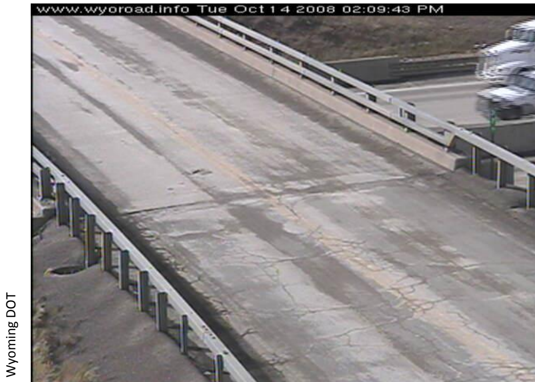
Figure 13. Icy Road Surface on Bridge near I-80 Summit
