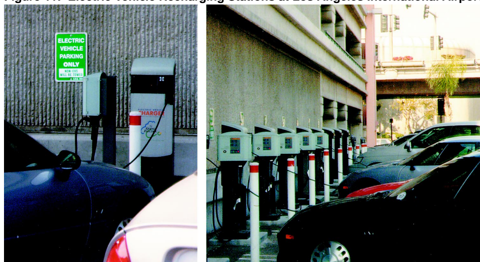
Figure 11: Electric Vehicle Recharging Stations at Los Angeles International Airport
