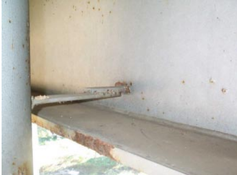
Figure 137. Localized corrosion on flange and web near the drain-to-girder web connection.
