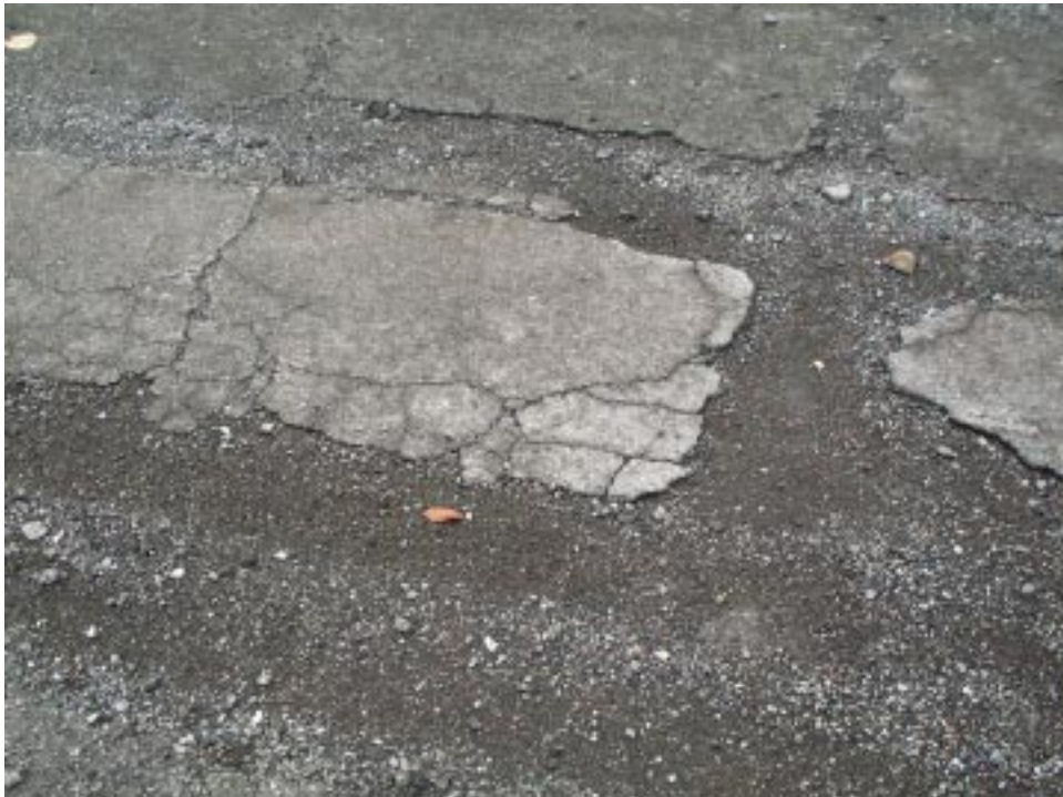
Figure 110. Deterioration described by Note B1 – Severe deterioration of wearing surface.
