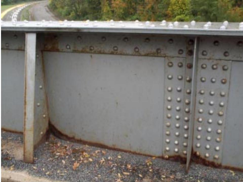
Figure 107. Deterioration described by Note A3 – Minor to moderate corrosion of stringer web at deck interface.
