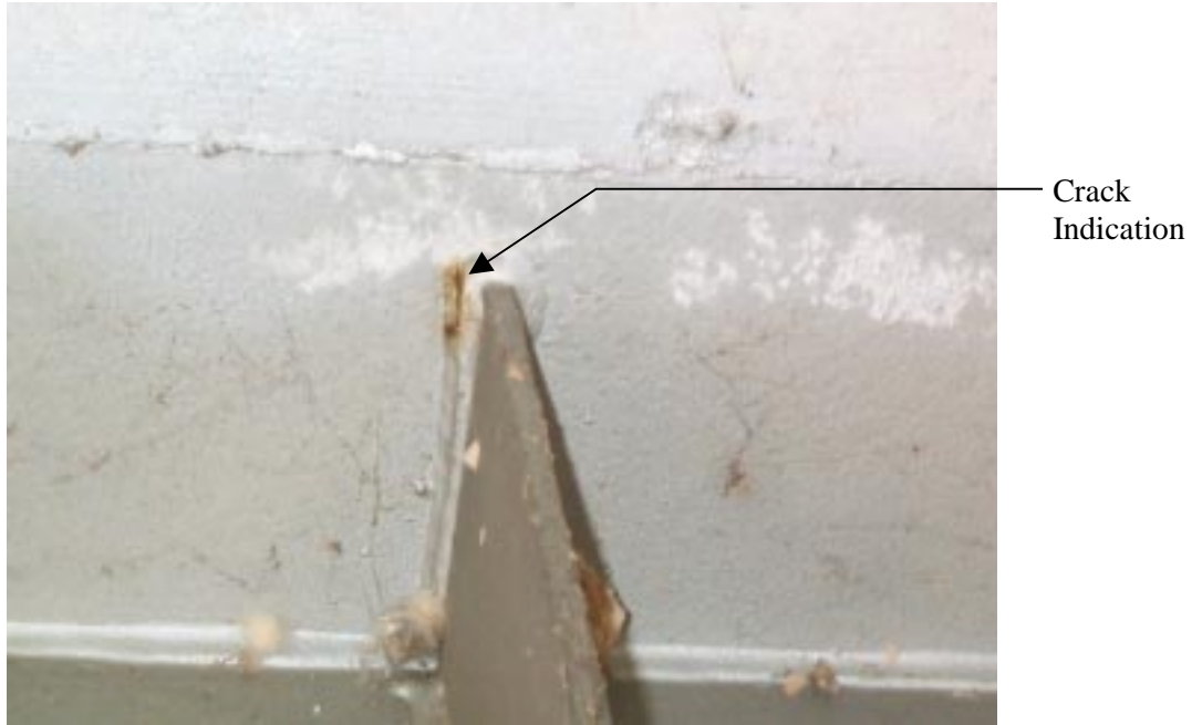
Figure 143. Weld crack indication W3 at vertical stiffener-to-top flange connection.
