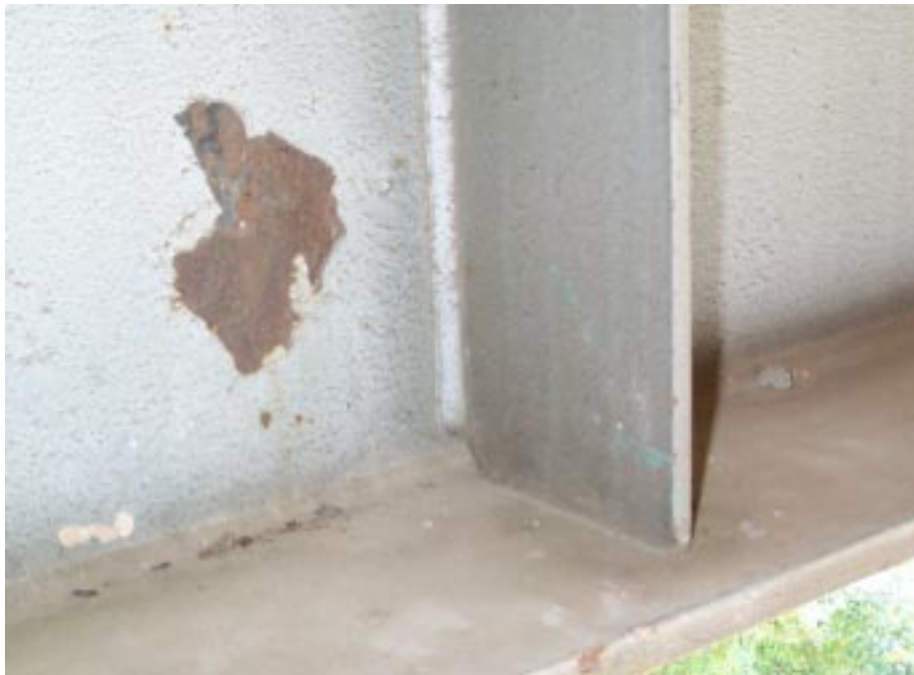
Figure 136. Paint failure on girder web.
