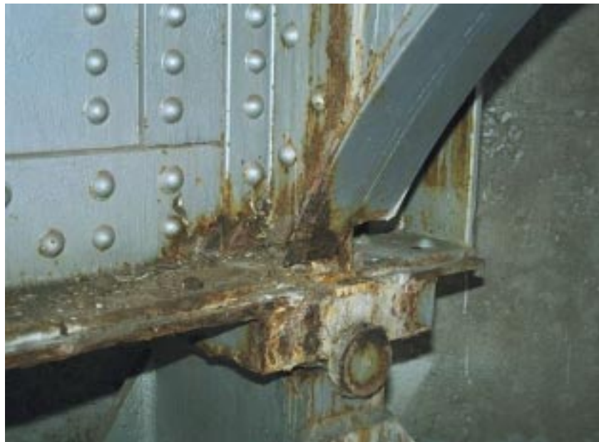
Figure 127. Paint system failure and moderate to severe corrosion.
