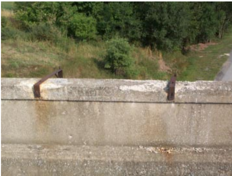
Figure 92. Inspector Photograph 6 – Failed overhead sign connection.
