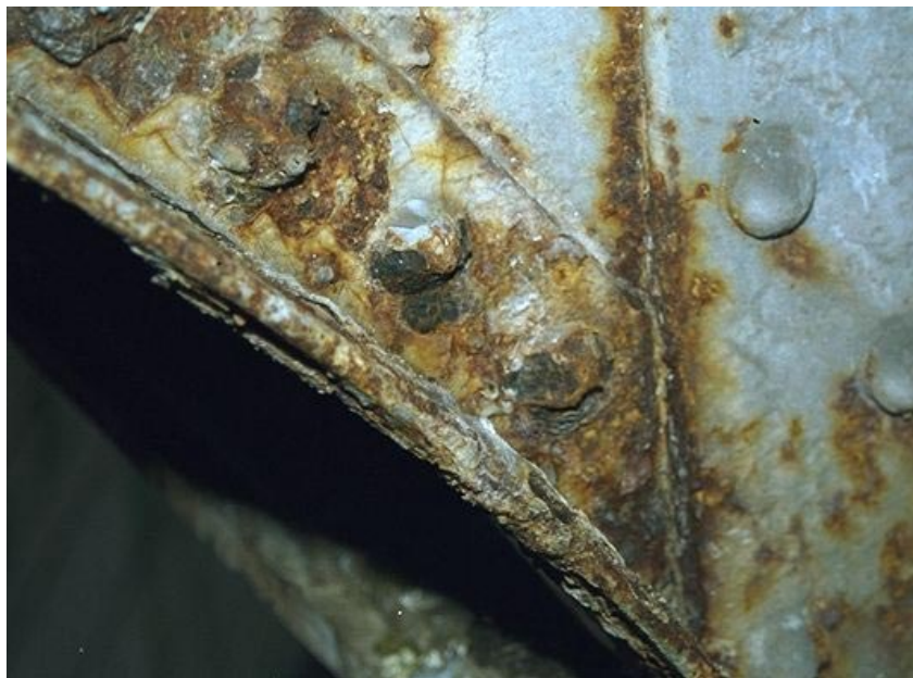
Figure 128. Severe corrosion of rivet heads.
