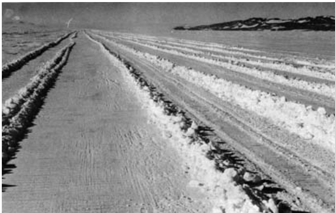
Figure 67. Windrows at the McMurdo Pegasus site. To prepare the snow-on-ice runway, the ice surface was scraped by heavy, long-track bulldozers and the well-mixed snow from the windrows was respread, compacted and graded. (Photo by M. Mellor, January 1990.)
