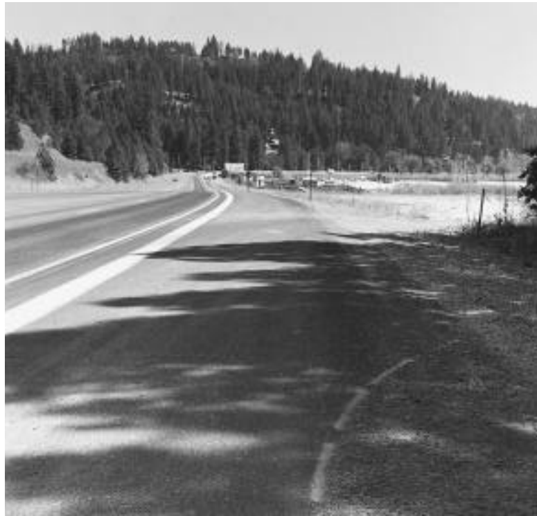
Federal highway project funds will convert this former route of Interstate 90 into a multi-use separated pathway.
