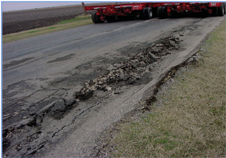
This photo, courtesy of the Texas Transportation Institute, shows pavement damage caused by heavy vehicles during spring thaw.
