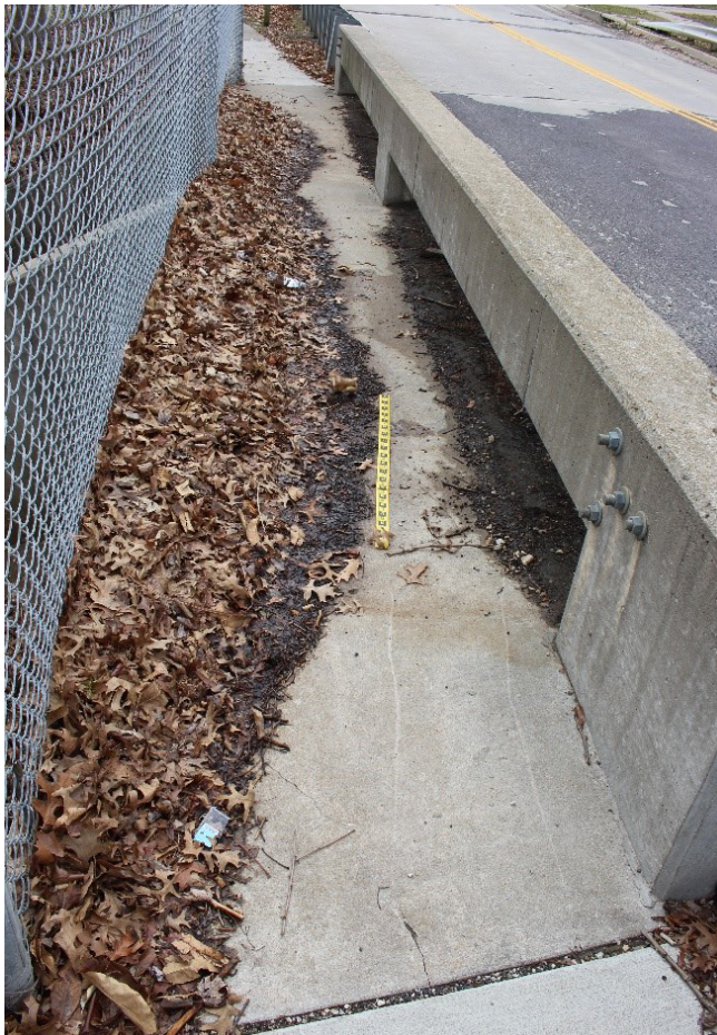
Debris accumulation that can cause corrosion and spalling
