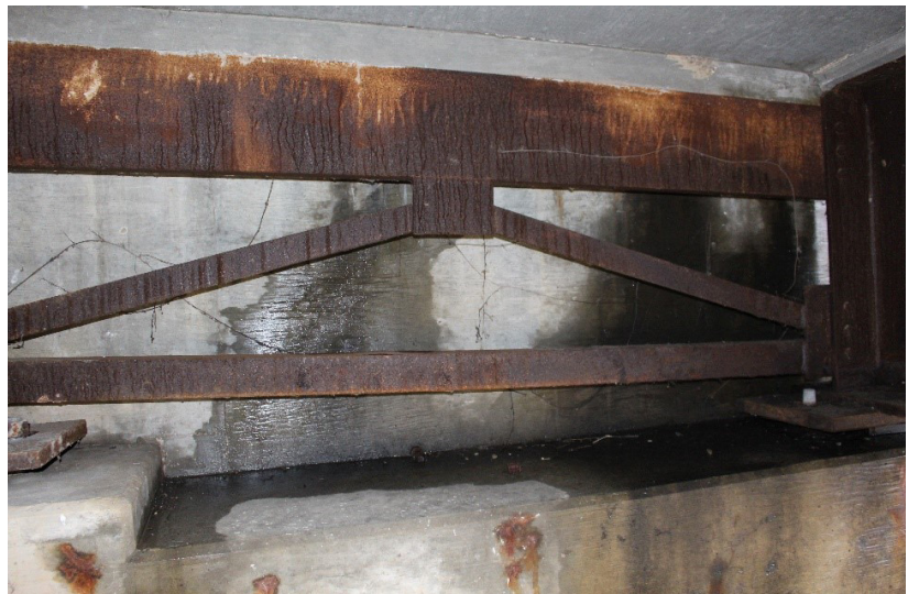
Corrosion damage caused by a leaking joint
