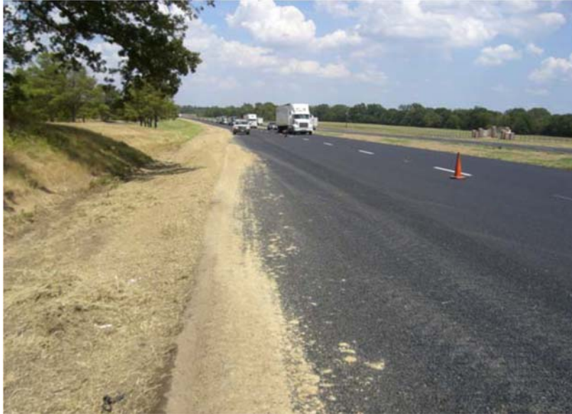
Figure 10. Clogging (Estakhri et al. 2008)
