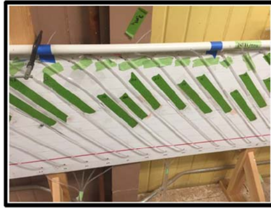
b) Manometer Board
