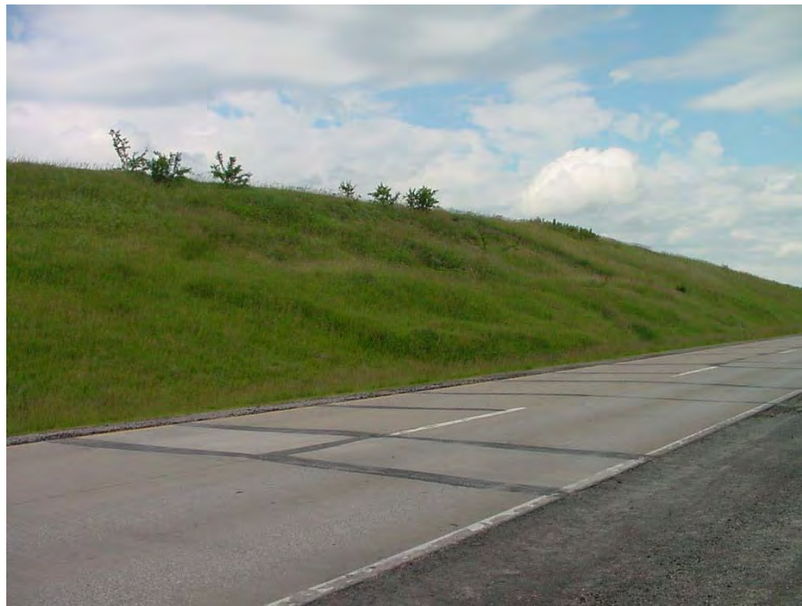
Figure 8.2 Photograph of US36-Stewartsville site taken after the recent slide at the site.
