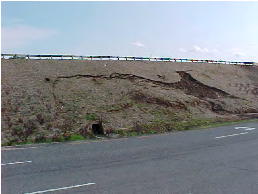
Figure 7.2 Photograph of most recent slide at I435-Wornall Road test site, June 20, 2001.
