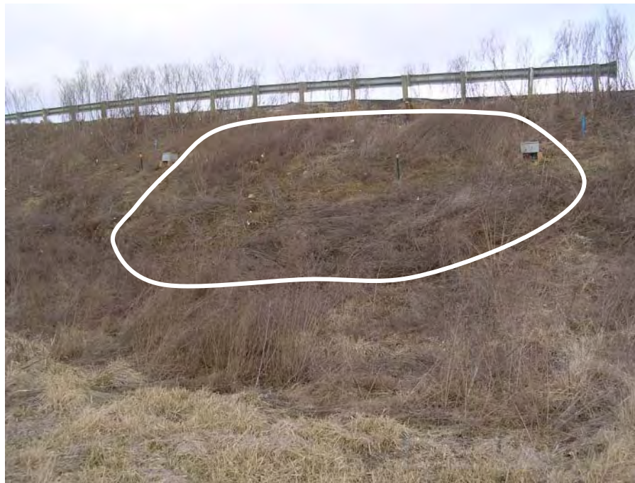
Figure 6.23 Observed failure in slide area S3 at I70-Emma site on January 27, 2005.
