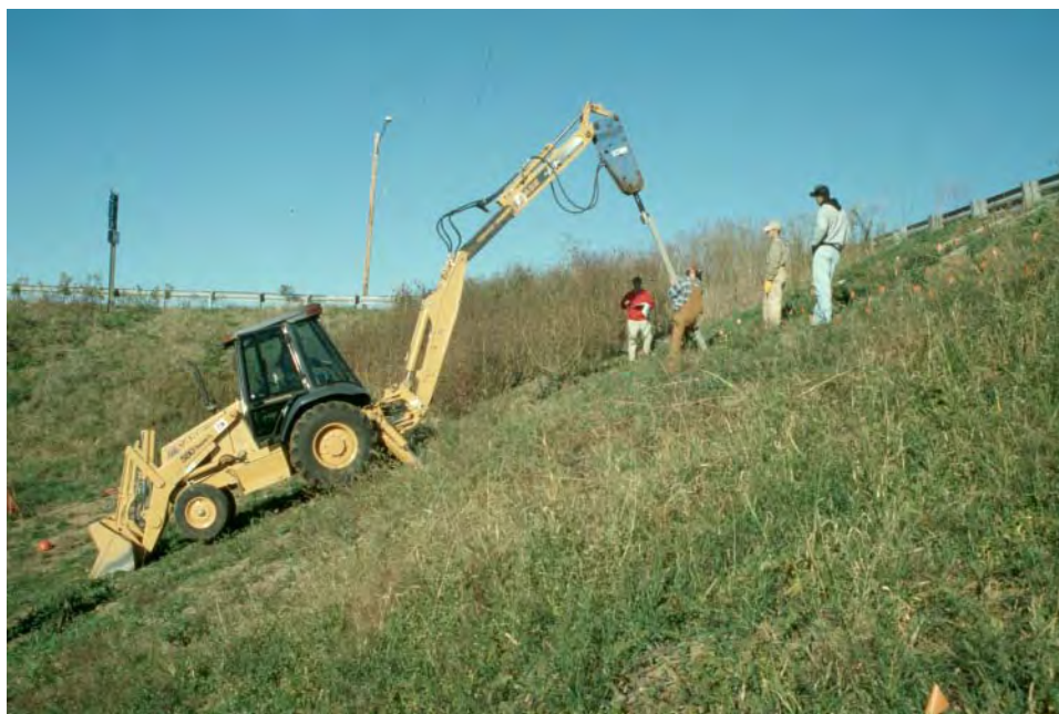
Figure 10.1 Backhoe mounted hammer used for initial installation attempts at the I70-Emma test site during Phase I.
