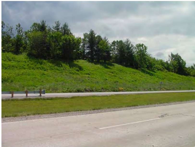
Figure 9.2 Photograph of US54-Fulton slope following most recent slide event.
