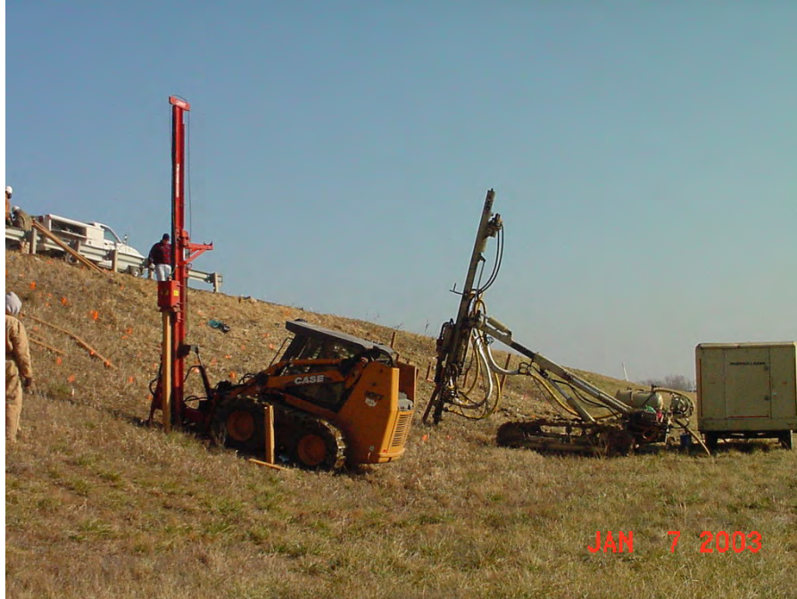
Figure 10.5 Ingersoll Rand ECM350 pneumatic hammer drill (background) and drop-weight hammer rig (foreground) used to install reinforcing members in slide area S3 at the I70-Emma site.
