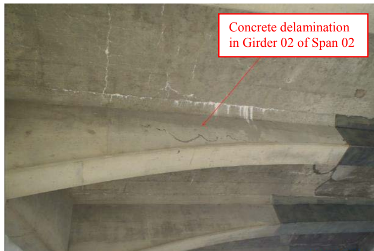
Figure 15 New Crack in Girder 02 Observed in November 2015
