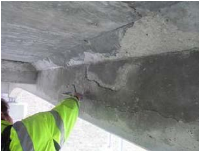
Figure 4 Typical Cracking Observed on All Four Beams
