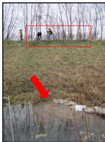
Figure 2-4 - The arrow indicates the location of a sand boil near the landside levee toe and the box indicates subsidence in levee crest due to loss of soil (Rutherford et al., 2016)
