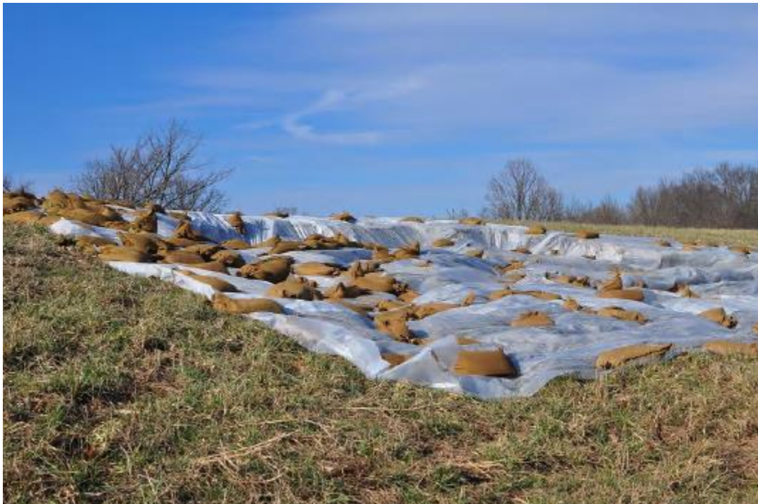
Figure 2-10 -Surface slide covered with plastic liner and sandbags near Grand Tower, IL (Rutherford et al., 2016)
