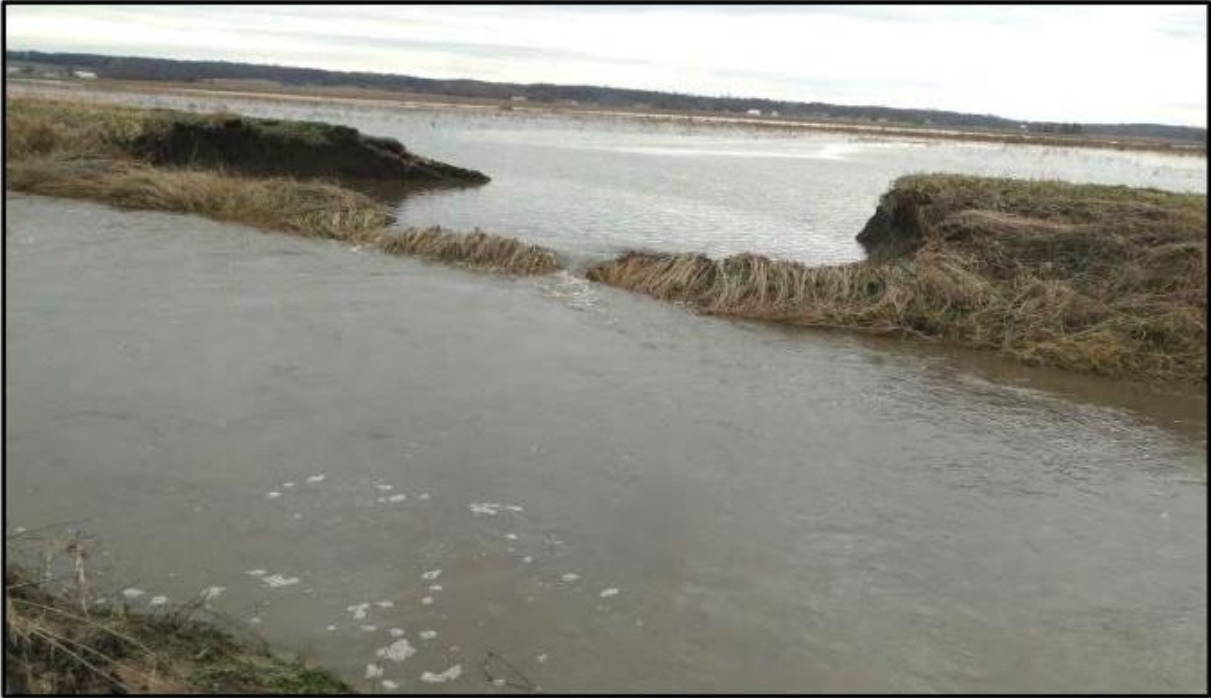
Figure 2-2 - overtopping erosion in a levee west of Oakford, IL (Rutherford et al., 2016)
