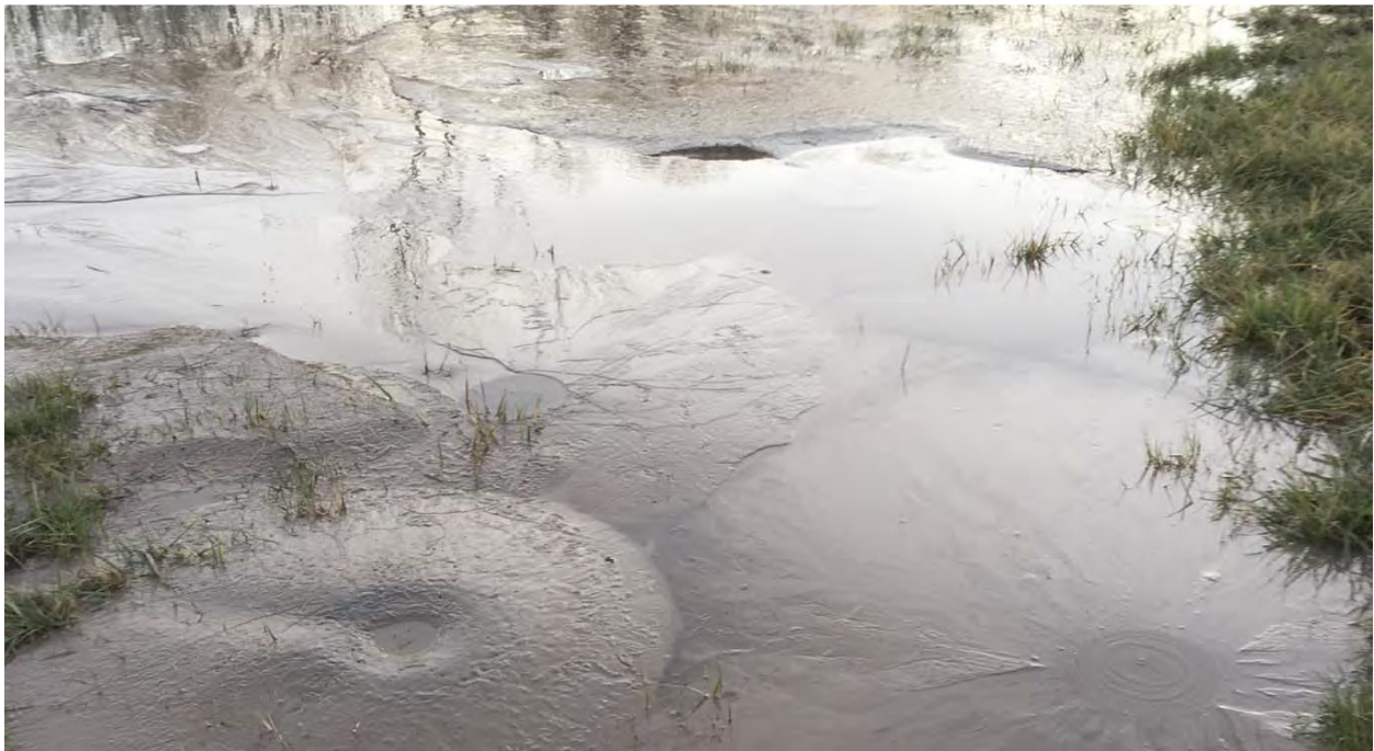
Figure 2-7 - Sand boils approximately 1,200 feet landward of the levee with water still seeping through near Cairo, IL (Rutherford et al., 2016)
