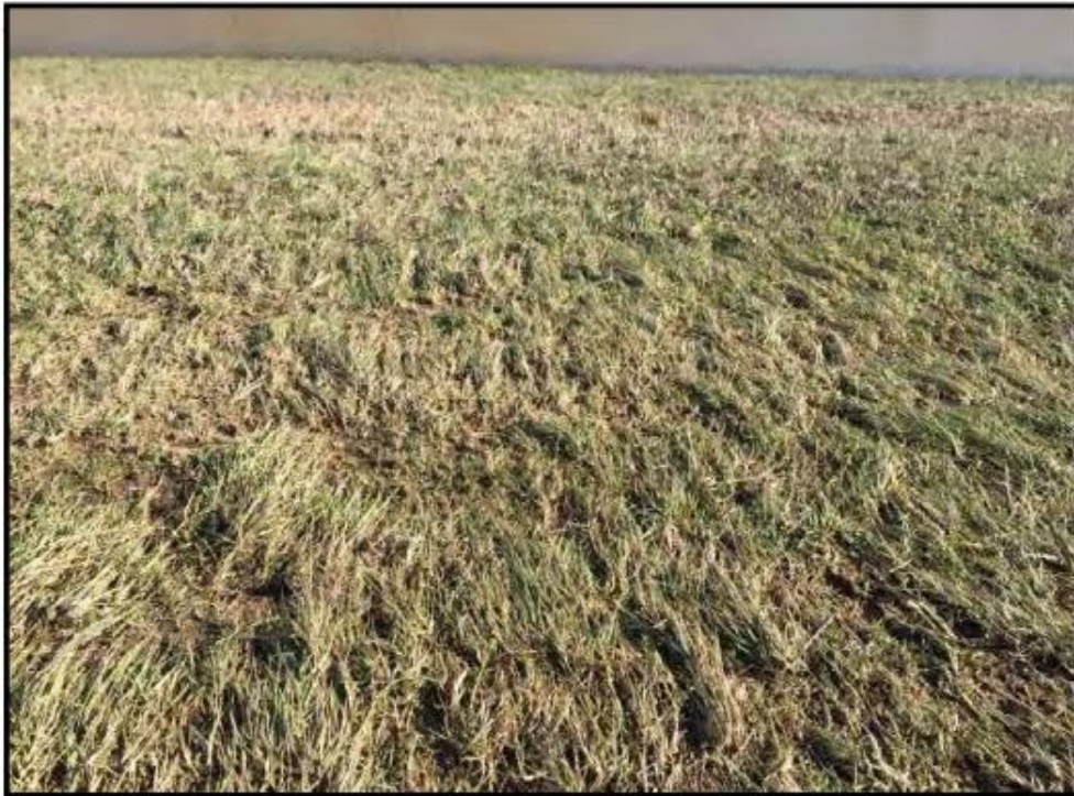
Figure 2-3 - vegetative cover laid down and acting as an armor on the landside slope of the levee near Olive Branch, IL (Rutherford et al., 2016)
