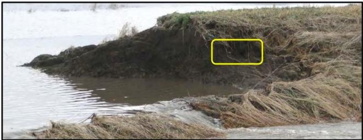
Figure 2-5 – View looking at exposed western edge of breach in a levee revealing the presence of animal burrows within the levee (Rutherford et al., 2016)
