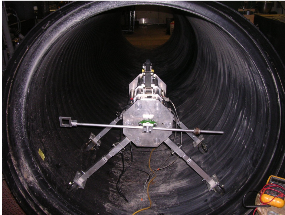
Figure 7. ORITE pipe crawler with laser profiler.
