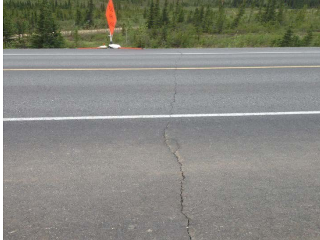
Figure 4.20 Natural transverse crack observed
