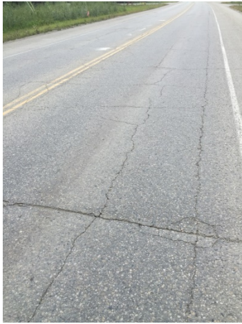
(a) Block cracks
