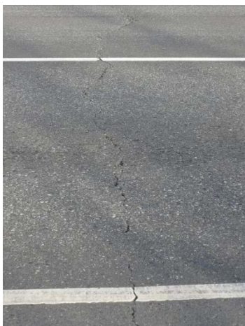
(a) Natural cracks
