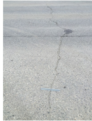
(c) Transverse crack
