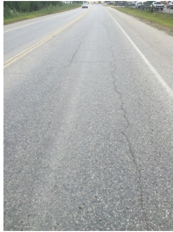
(b) Longitudinal crack
