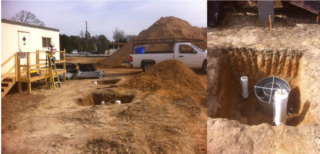
Figure 7. Two test pits located at the Lawrenceville, GA site are shown. A test set up is also shown in one of the test pits
