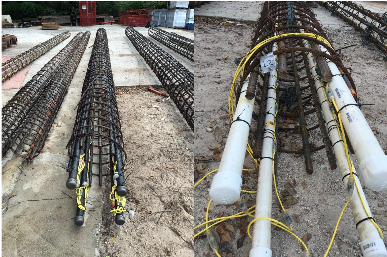
Figure 2.5 Bottom end view of reinforcement cages for 24-in piles C2 (left) and L2 (right) instrumented with thermal wires and access tubes for thermal probe testing.
