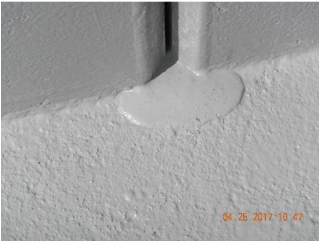
Figure 4 Pooled coating due to severe run (notice pin holing)
