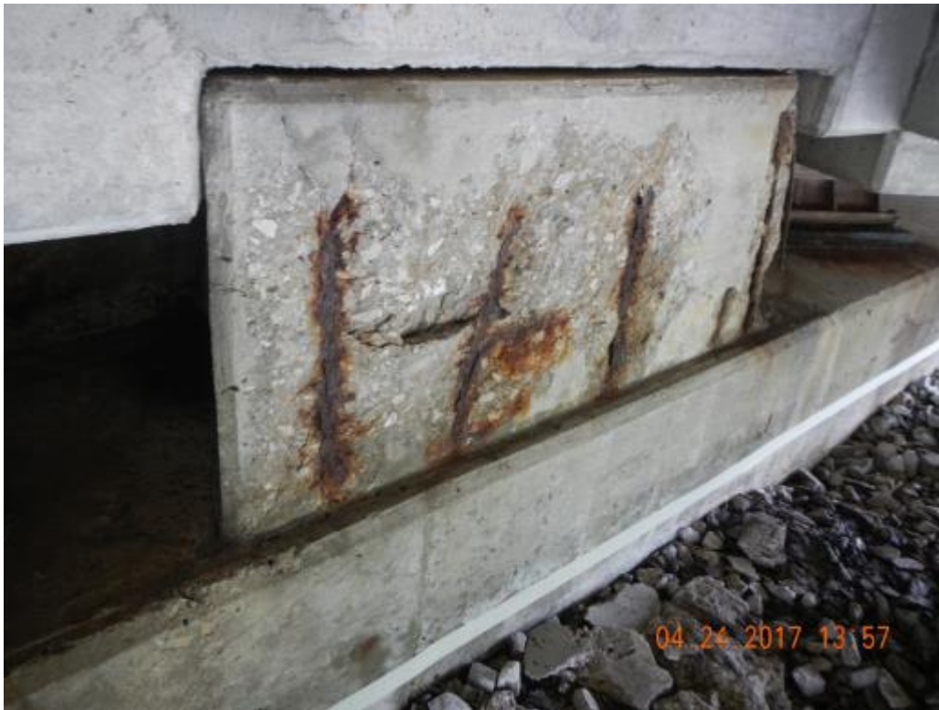
Figure 5 Spalled area on abutment after cleaning
