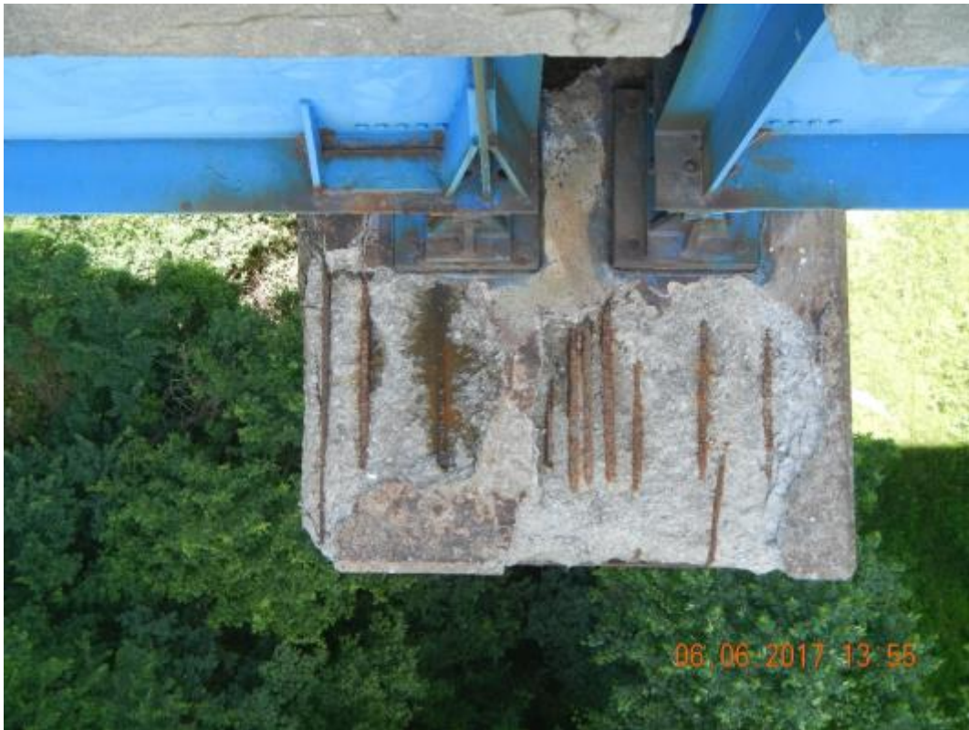
Figure 13 Pier cap with severe spalling (post washing)
