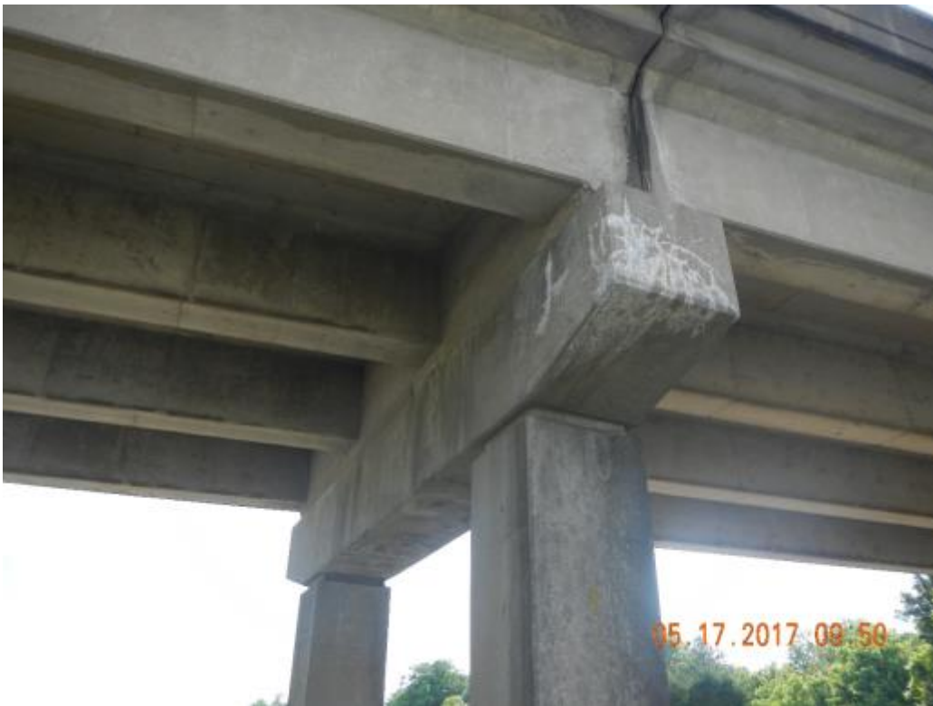
Figure 10 Efflorescence on pier cap after cleaning
