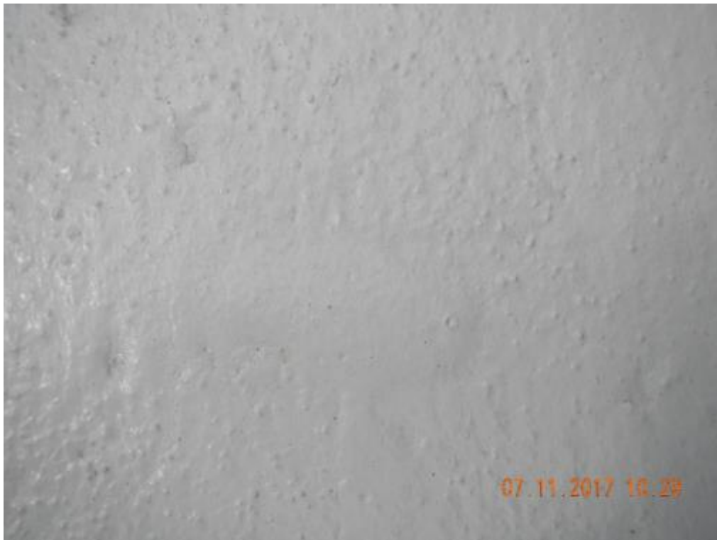
Figure 16 Pinholes due to thickness coating application
