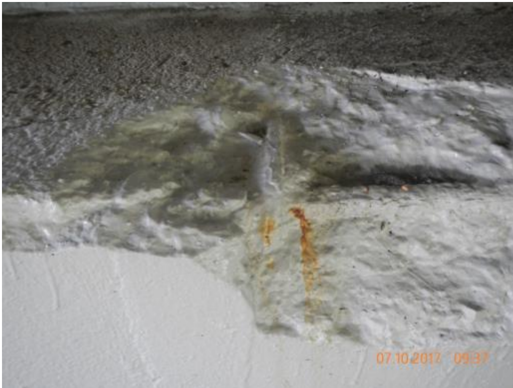
Figure 15 Unrepaired spalling with exposed reinforcement 12 weeks after coating
