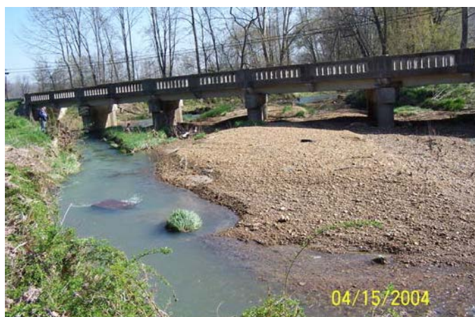
Figure 34. Loose Rock and Sediment Deposits at KYTC Bridge
