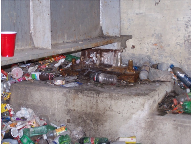
Figure 14. Trash Build-Up on a Bridge Abutment
