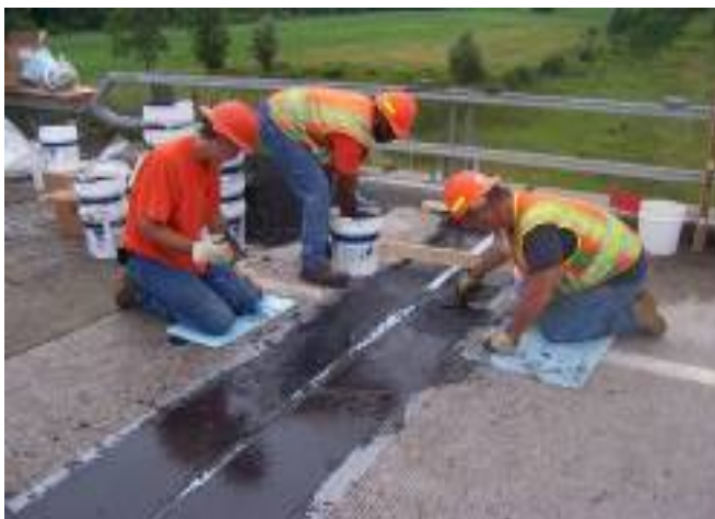
Figure 2. Installation of a Blockout Prior to Seal Installation. Foam stripping between the blockouts acts as a form and controls joint opening size.
