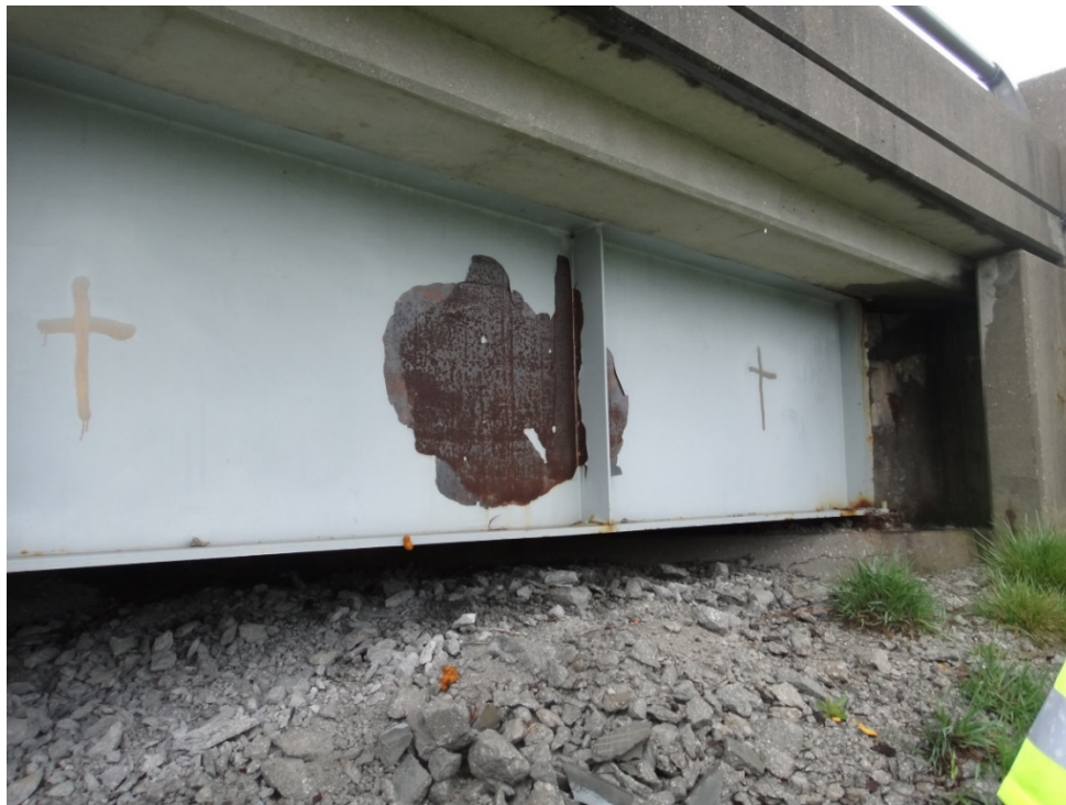
Figure 18. Spot Coating Failure
