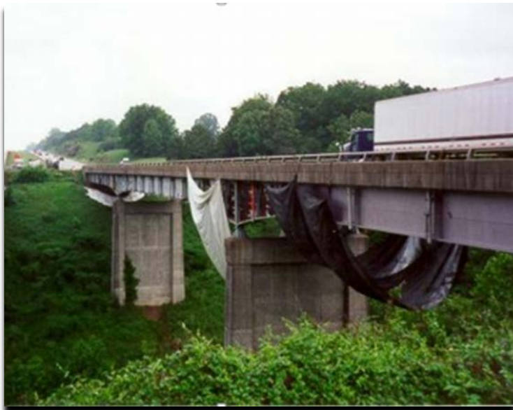
Figure 19. Diaper Placed Under a Bridge to Catch Paint Debris
