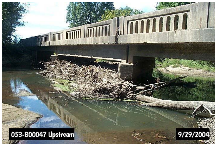
Figure 33. Drift Trapped at KYTC Bridge
