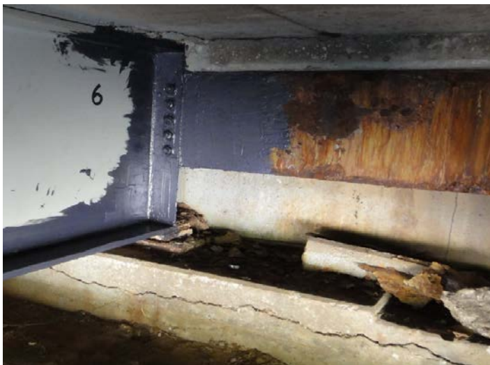
Figure 30. Abutment Cap Cracked Due to Leaking Joint and Deicing Chemical Damage
