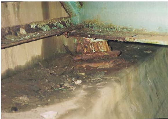
Figure 12. Tilted Rocker Bearing Requiring Cleaning and Resetting (14)
