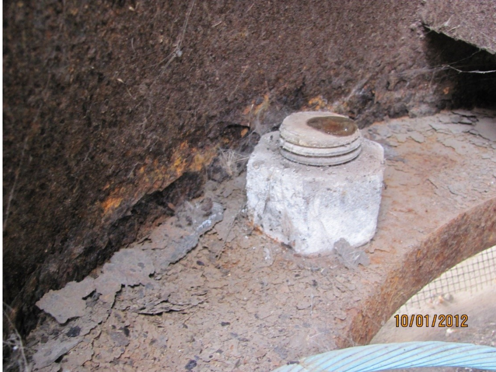
Figure 4.9 Duluth High Mast Light Interior Corrosion Photo.
