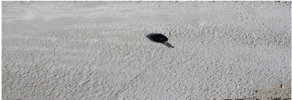
Figure 39: Photograph of fiber reinforced LMC overlays after 165 days.
