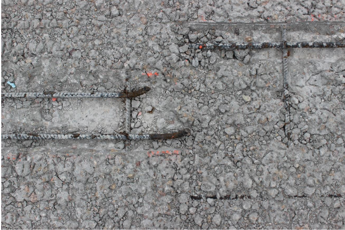
Figure 42: Photograph of scarification in the pour-site (quarter span).
