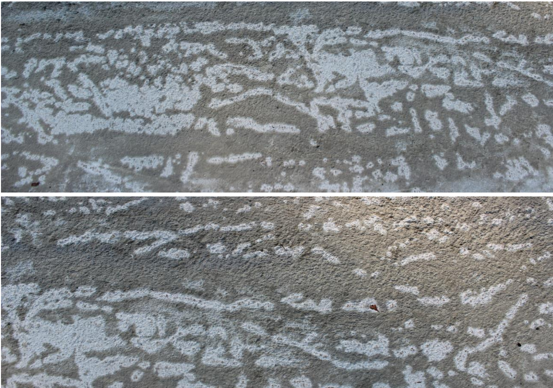
Figure 27: Photograph of fiber reinforced LMC overlays after 1 day.
