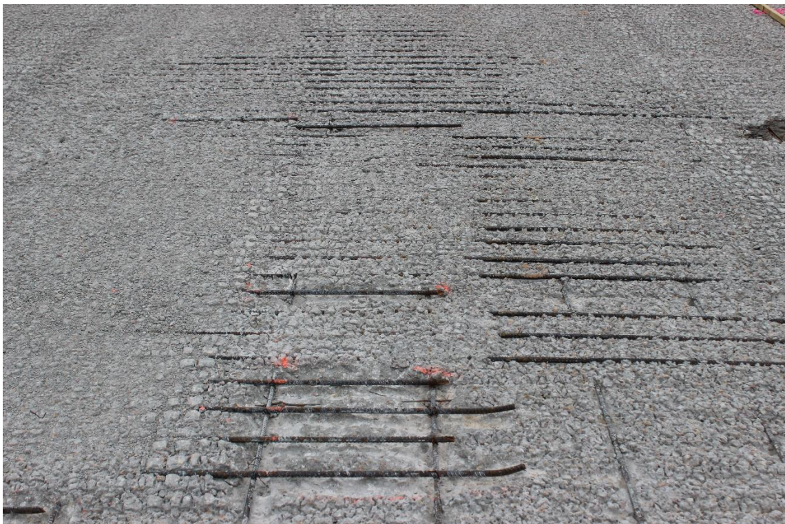
Figure 43: Photograph of scarification on bridge opposite of the pour site.
