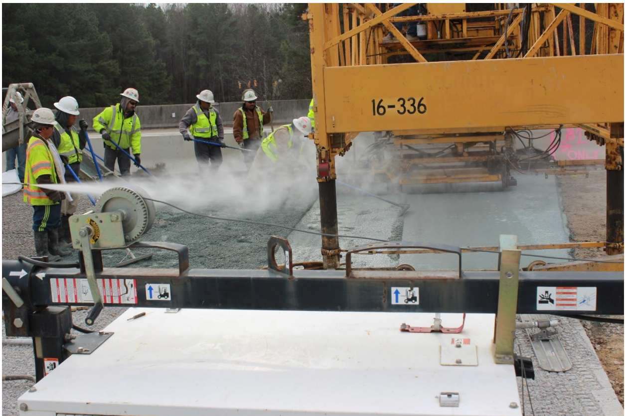
Figure 49: Spraying of water over the fresh concrete via a pressurized water sprayer.
