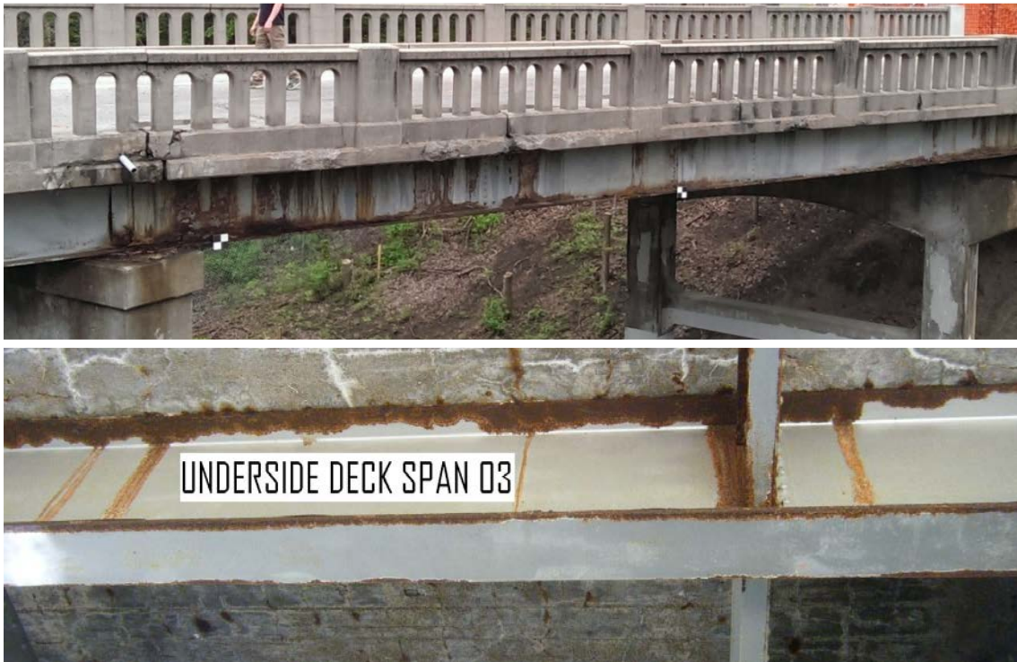
Figure 3.3 Deterioration pattern where entire section of girder is deteriorated
