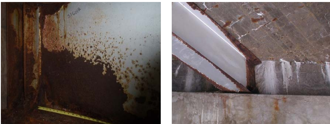
Figure 3.1 Deterioration pattern at girder ends
