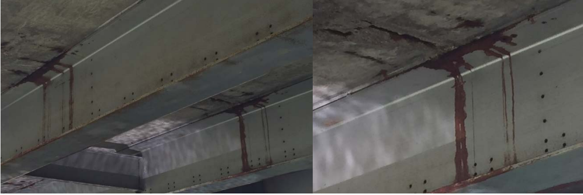
Figure 3.4 Entire girder section deteriorated below the cracked slab
