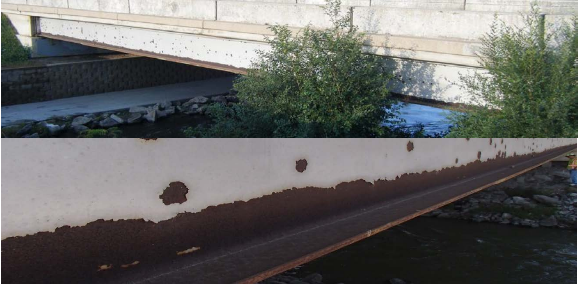
Figure 3.2 Bottom flange deterioration along the girder
