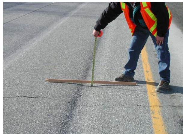
Studded Tire Damage (wear) to HMA in Washington State (TRB 09-2205 pg. 4)
