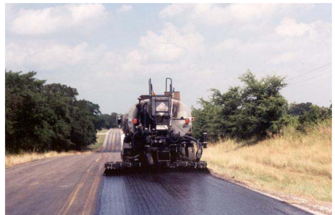
Non-uniform binder application can cause streaking.
