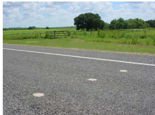
Southbound Lane Sand Circles on Highway 19 (TRB 09-0411 pg. 5)
