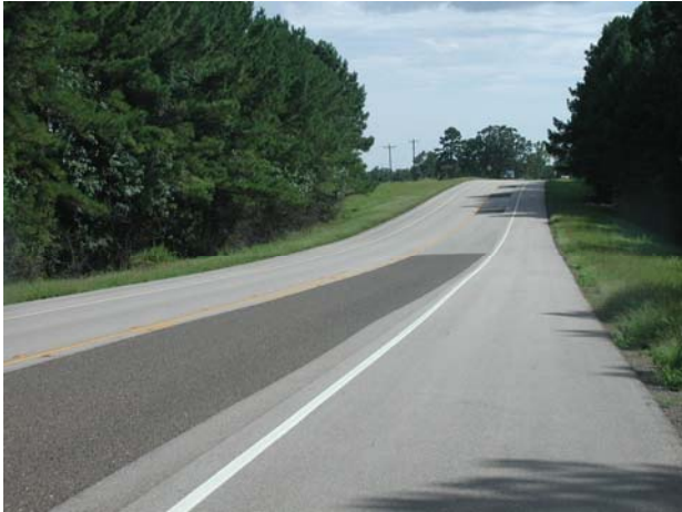
A typical strip seal coat covers the right-hand lane of this road.
